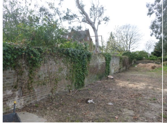
12. Mortared wall with sparse ivy cover (U1e - 68)
