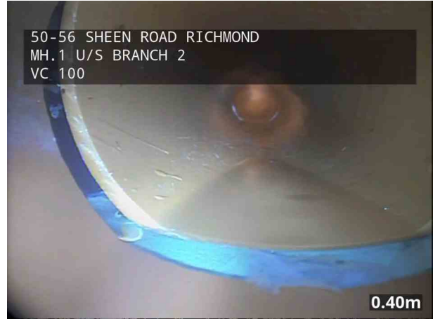
_50-56 SHEEN ROAD_RICHMOND_2_004.jpg, 00:00:00, 0.40 m Joint displaced, medium
