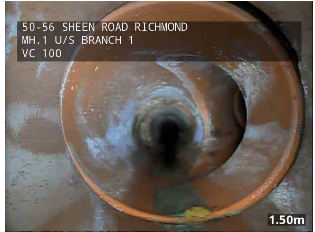
50-56 SHEEN ROAD RICHMOND MH.1 U/S BRANCH 1 VC 100 1.50m _50-56 SHEEN ROAD_RICHMOND_1_002.jpg, 00:00:09, 1.50 m Joint displaced, medium
