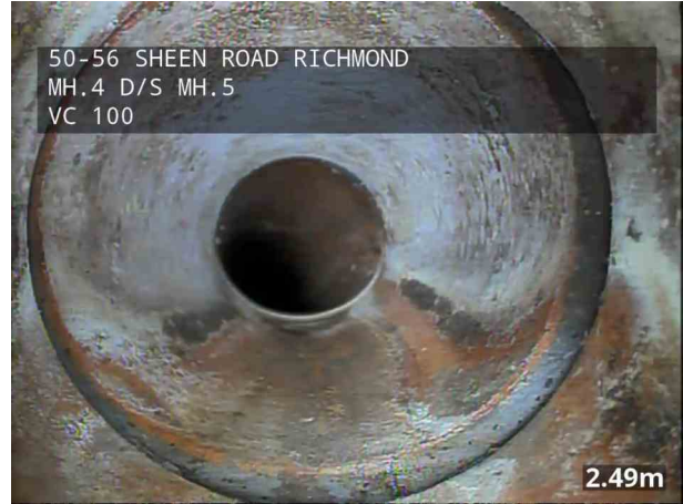
50-56 SHEEN ROAD_RICHMOND MH.4 D/S MH.5 VC 100 2.49m _50-56 SHEEN ROAD_RICHMOND_11_017.jpg, 00:00:11, 2.49 m Joint displaced, medium
