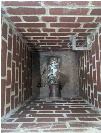
_50-56 SHEEN ROAD_RICHMOND_11_018.jpg, 00:00:22, 4.47 m Finish node, manhole, reference: MH.5, DEBRIS IN
