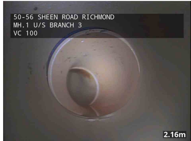
_50-56 SHEEN ROAD_RICHMOND_3_006.jpg, 00:00:11, 2.16 m Joint displaced, medium
