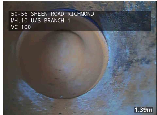
50-56 SHEEN ROAD RICHMOND MH.10 U/S BRANCH 1 VC 100 1.39m _50-56 SHEEN ROAD_RICHMOND_25_036.jpg, 00:00:08, 1.39 m Joint displaced, medium
