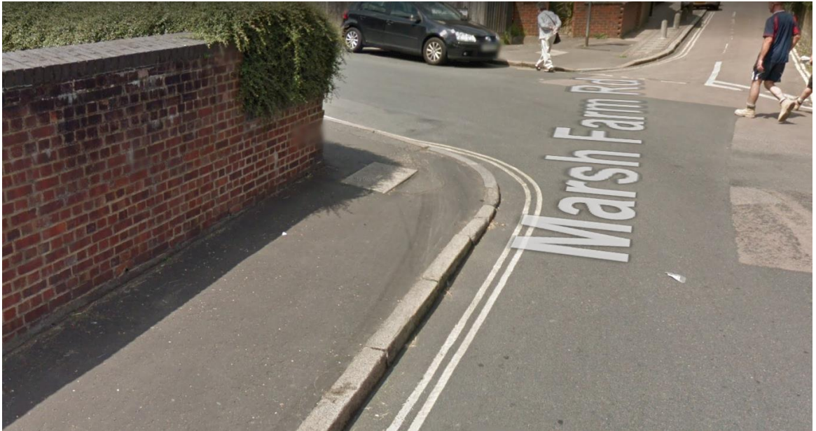
Figure 1-3: Tyre marks on Marsh Farm Road footway
