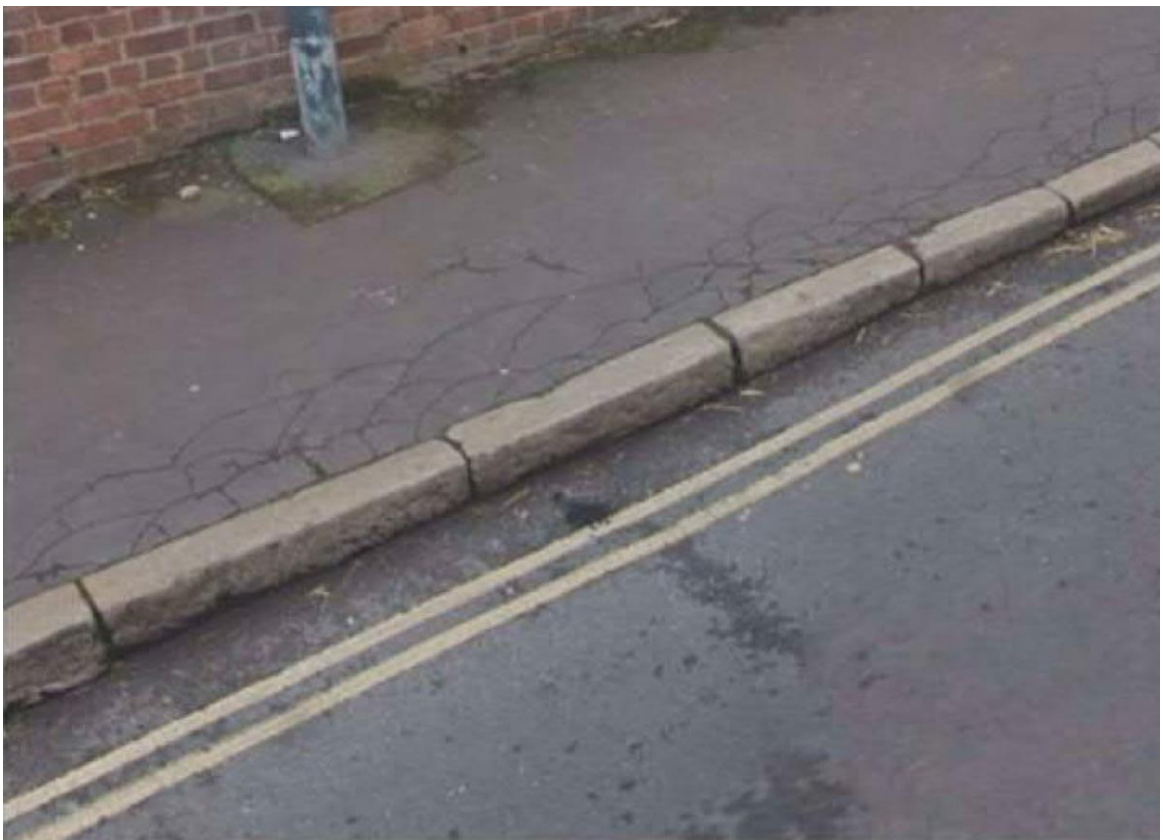
Figure 1-2: Damage to Marsh Farm Road footway
