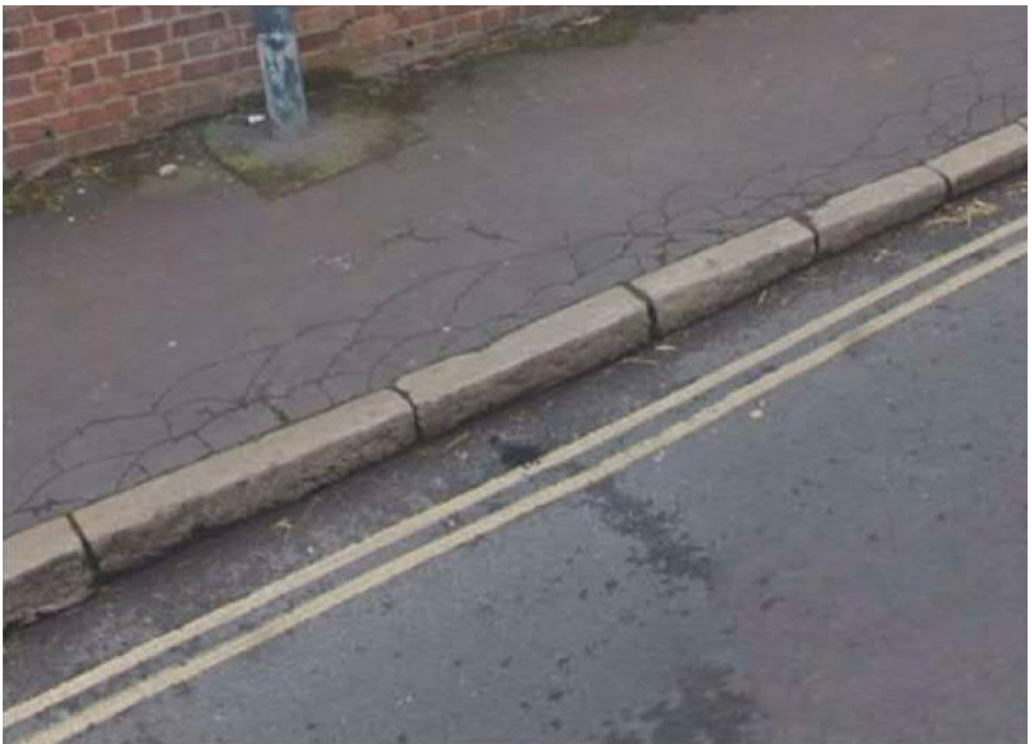
Figure 1-2: Damage to Marsh Farm Road footway
