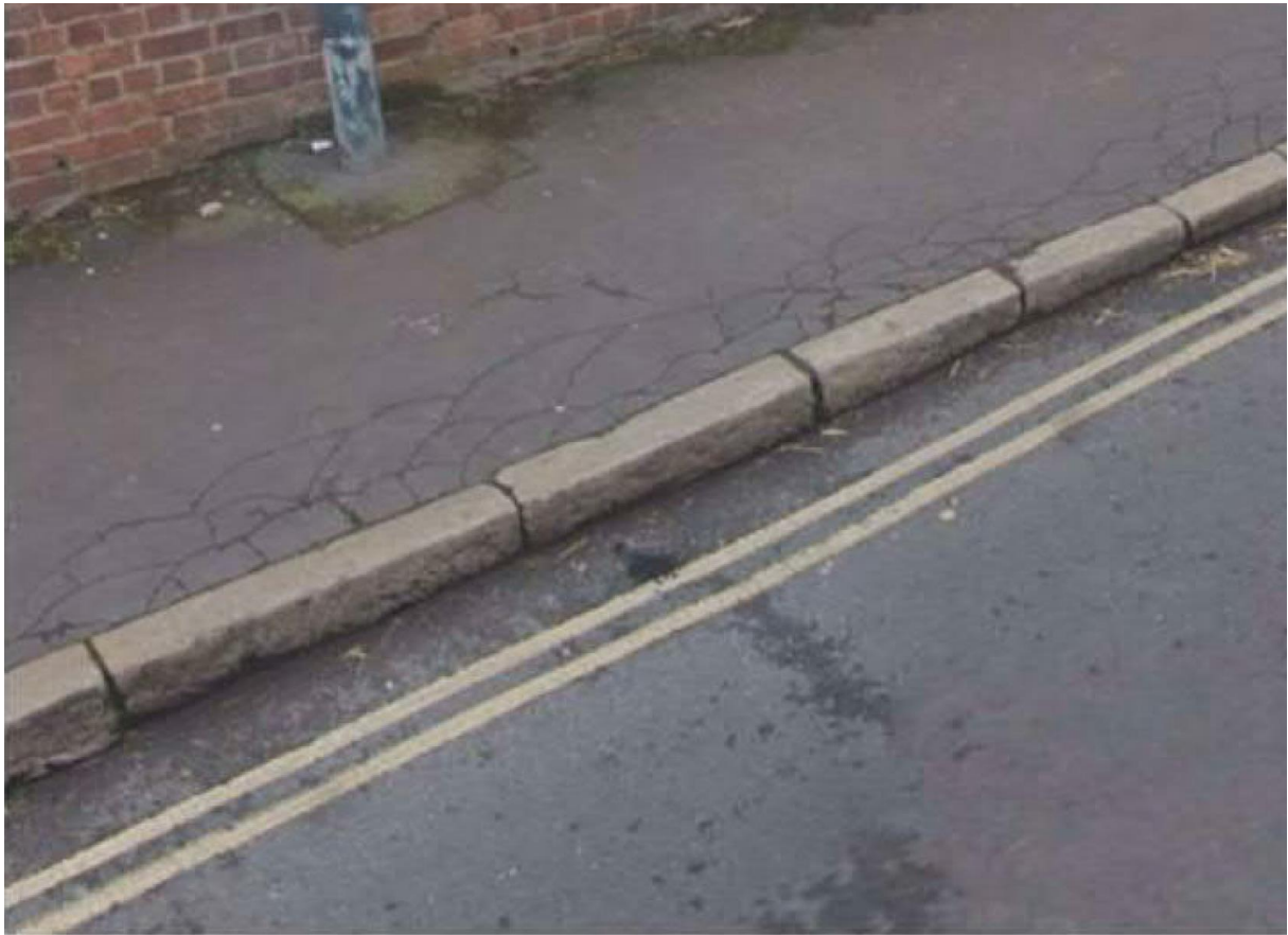
Photo 2: Damage to Marsh Farm Lane footway from vehicles mouting the kerb
