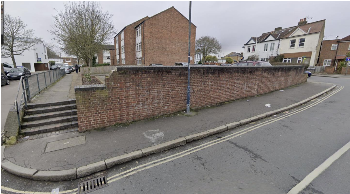
Photo 4: Damage to Marsh Farm Lane footway from vehicles mouting the kerb
