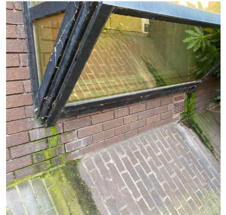
2. Current Building Envelope Condition - Condensation & Moss caused by the existing cladding detail
