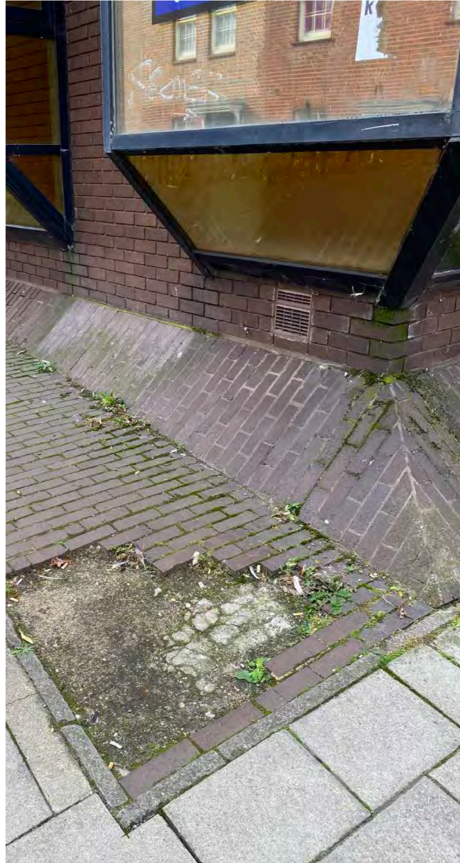
4. Missing Pavers in Public Realm
