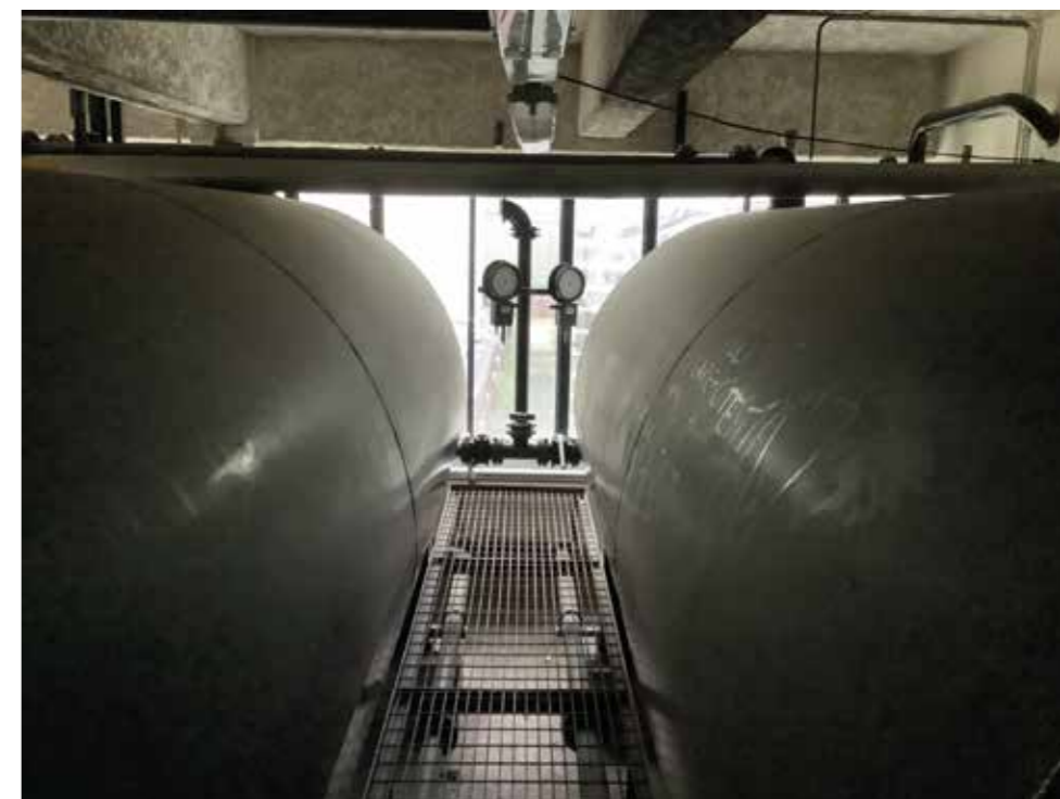
Residual former Dilac tanks at west site, empty but not yet removed
