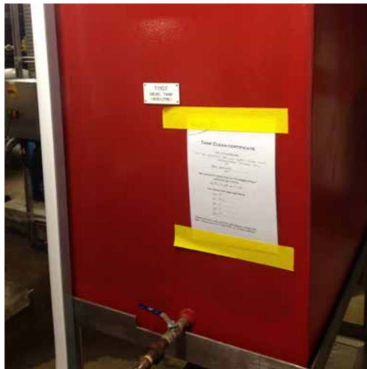
Decommissioned diesel tank in Production Office basement
