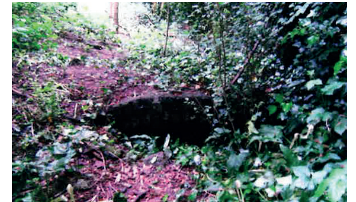
Refer to Whitton Brook -A Small River Journey Through Whitton History by Ed Harris- Page 20 19th Century Brick Culvert found North of Cambridge Close, has been completely dry for centuries.
