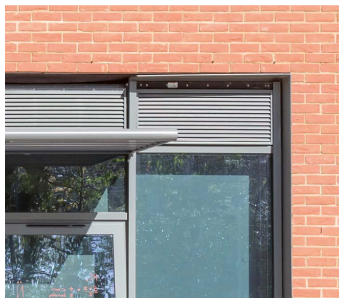
An image of the louvres which sit in front of the MVHR units at the top of the window
