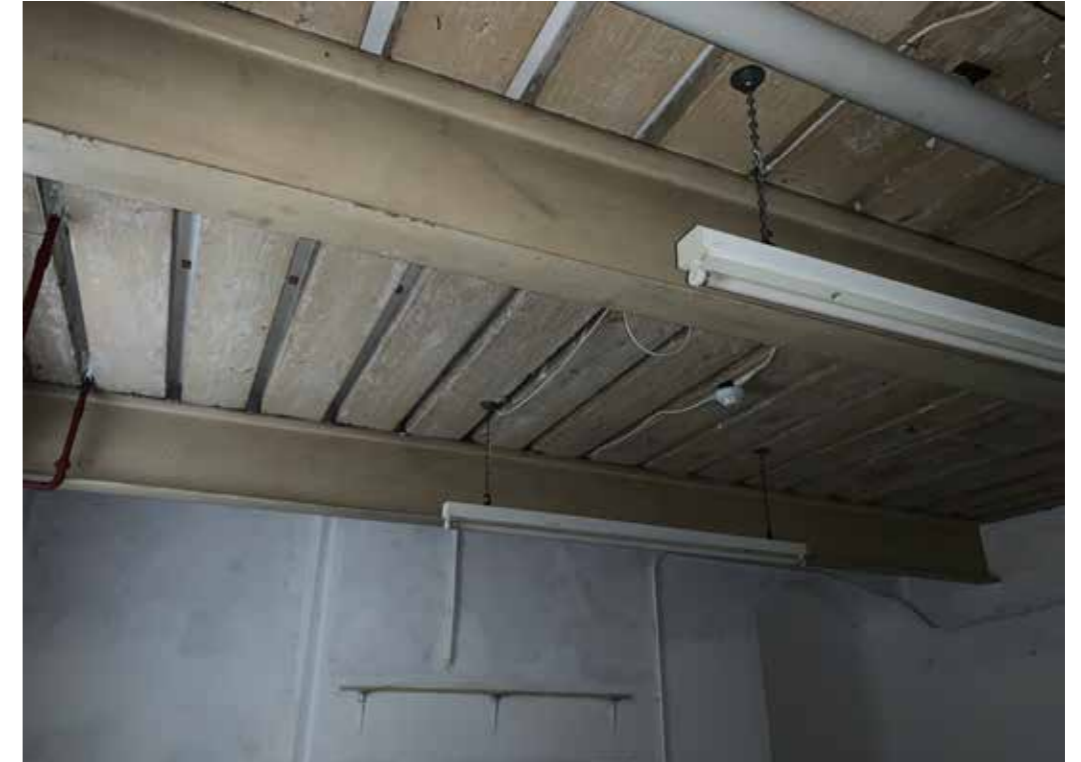
Figure 4.7 Modern ceiling beams and joists have been introduced in many rooms within the basement and replace historic features
