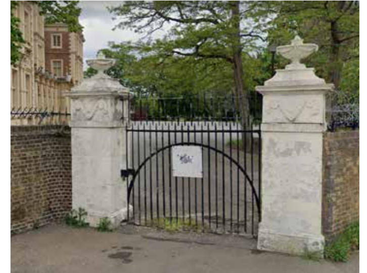
Figure 3.42 Photograph of a disused historic entrance with its pair of stone gate piers
