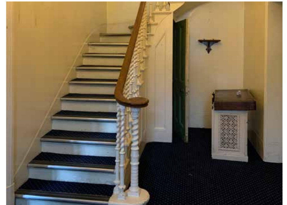
Figure 4.17 A historic staircase survives in the rear entrance hall. Modern carpet and nosings have been fitted to its treads and detract from its interest. Chasing in the plastered wall to the right indicates the historic location of an additional flight of stairs
