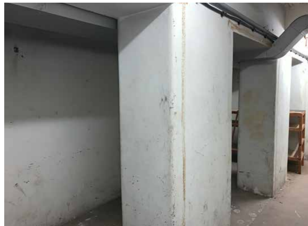
Figure 4.6 Early nineteenth-century supportive columns in the basement. Modern MEP equipment has been inappropriately fitted here.
