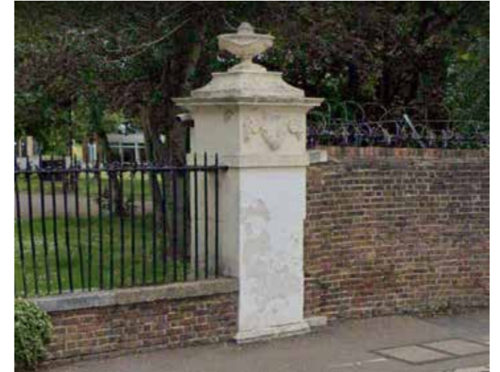
Figure 3.44 Photograph of a stone gate pier which marks the junction between the boundary wall and boundary railings
