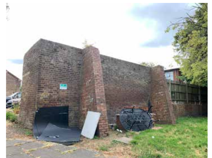
Figure 3.48 The rear elevation of the surviving section of garden wall, showing the modern buttressing. The south returning end of the wall (right) has been rebuilt using modern brick and fencing.
