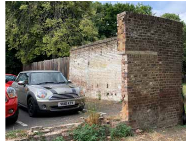
Figure 3.46 Photograph of the surviving section of garden wall. The wall is in a state of disrepair and is structurally unstable.
