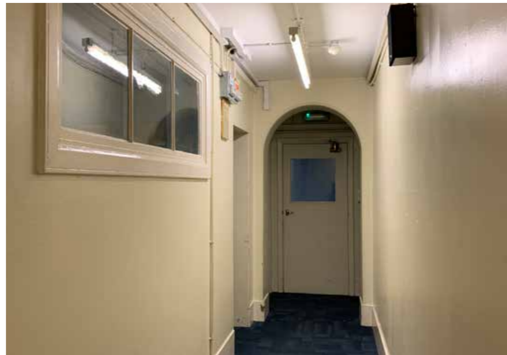
Figure 4.22 Historic arches located at either end of the rear corridor, located behind the chapel at second-floor level, provide a source of interest to the building
