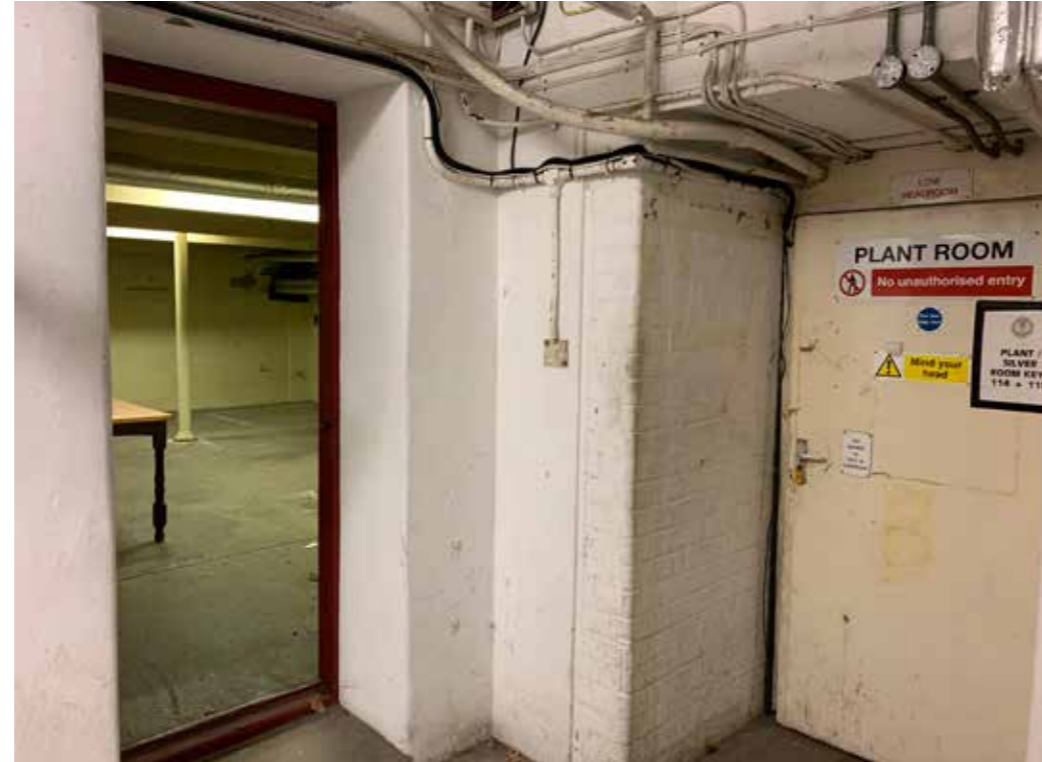
Figure 4.5 A typical corridor within the basement of the hall comprising early nineteenth-century walls which have been inappropriately fitted with exposed MEP equipment. Modern doors have also been introduced here.
