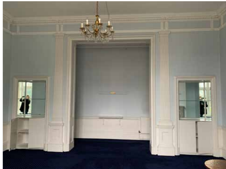
Figure 4.15 Openings in this wall, located behind the rear wall of the main entrance hall, have been infilled with modern cupboards. These features are considered to detract from the interest of the room
