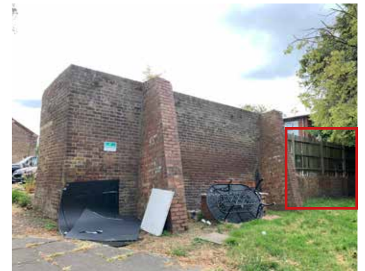
Figure 3.50 The rear elevation of the surviving section of garden wall, showing the modern buttressing. The south returning end of the wall (right) has been rebuilt using modern brick and fencing. This section of wall (also highlighted in red) will be rebuilt using material from the surviving north end of the wall
