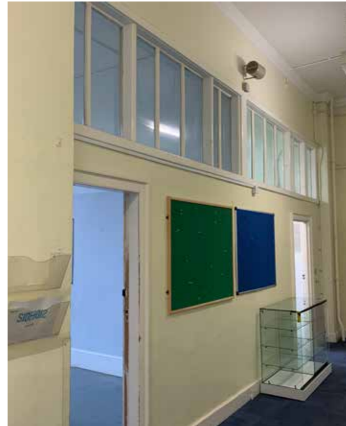
Figure 4.9 Detractive modern partition walls have been installed west of the main entrance hall. They comprise a plain design and have subdivided an historic classroom to create multiple rooms and a corridor
