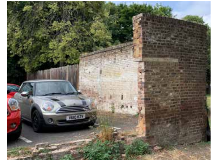
Figure 3.49 Photograph of the surviving section of garden wall. The wall is in a state of disrepair and is structurally unstable
