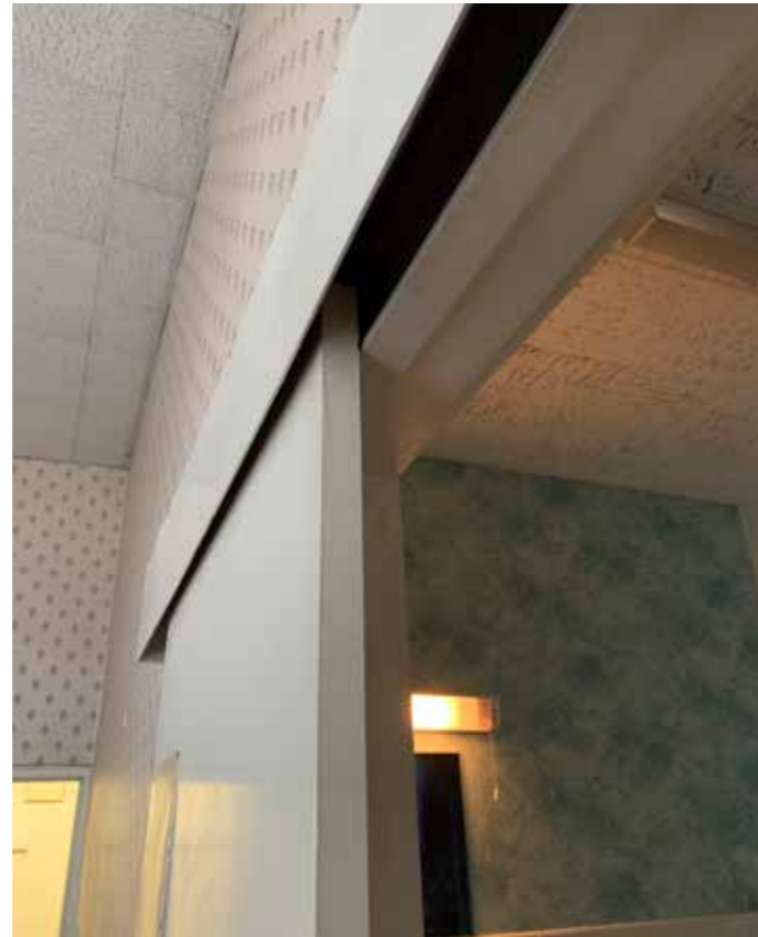
Figure 4.18 An example of the many modern partition walls introduced to subdivide historic spaces in the building. Modern dropped ceilings have also commonly been installed. The room in the photograph has been created through the subdivision of the former Vice Principal's bedroom and sitting room
