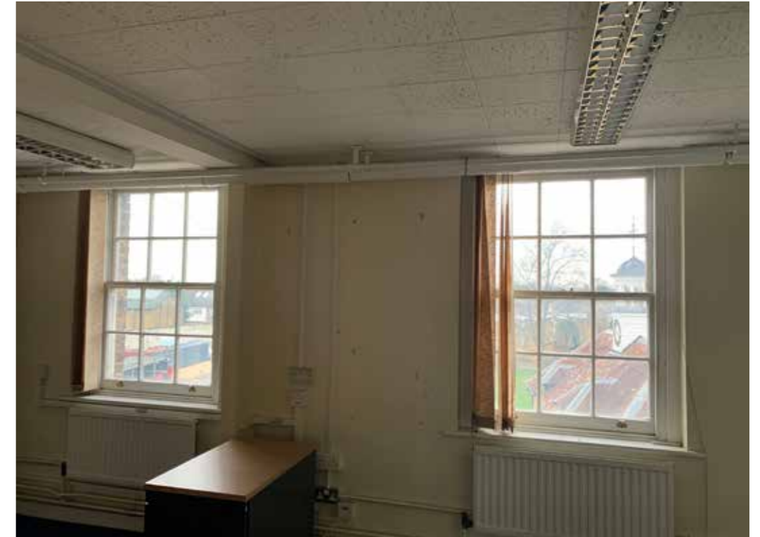
Figure 4.27 A typical modern dropped ceiling located within the west wing conceals the tops of historic windows and negatively alters the historic volume of the space
