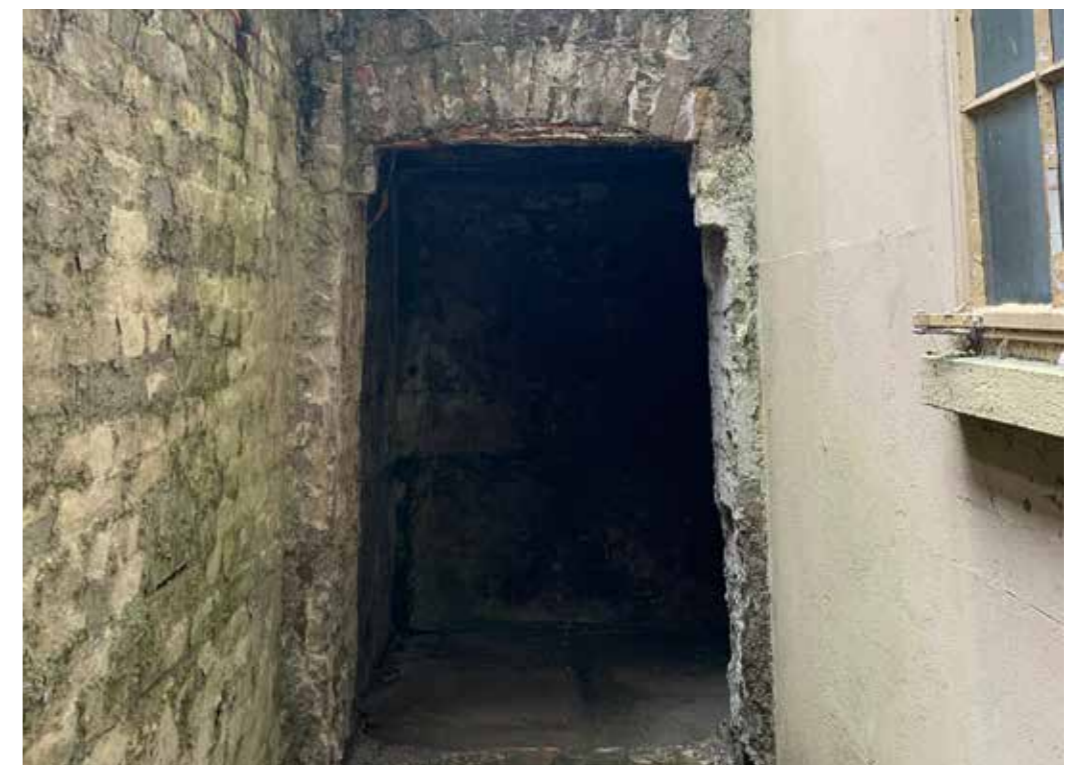
Figure 4.8 An historic external entrance survives at the rear of the basement but is in a state of disrepair
