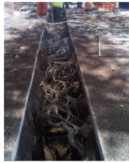
Example imagery of air spade use for implementing utilities beneath root plate (existing)
