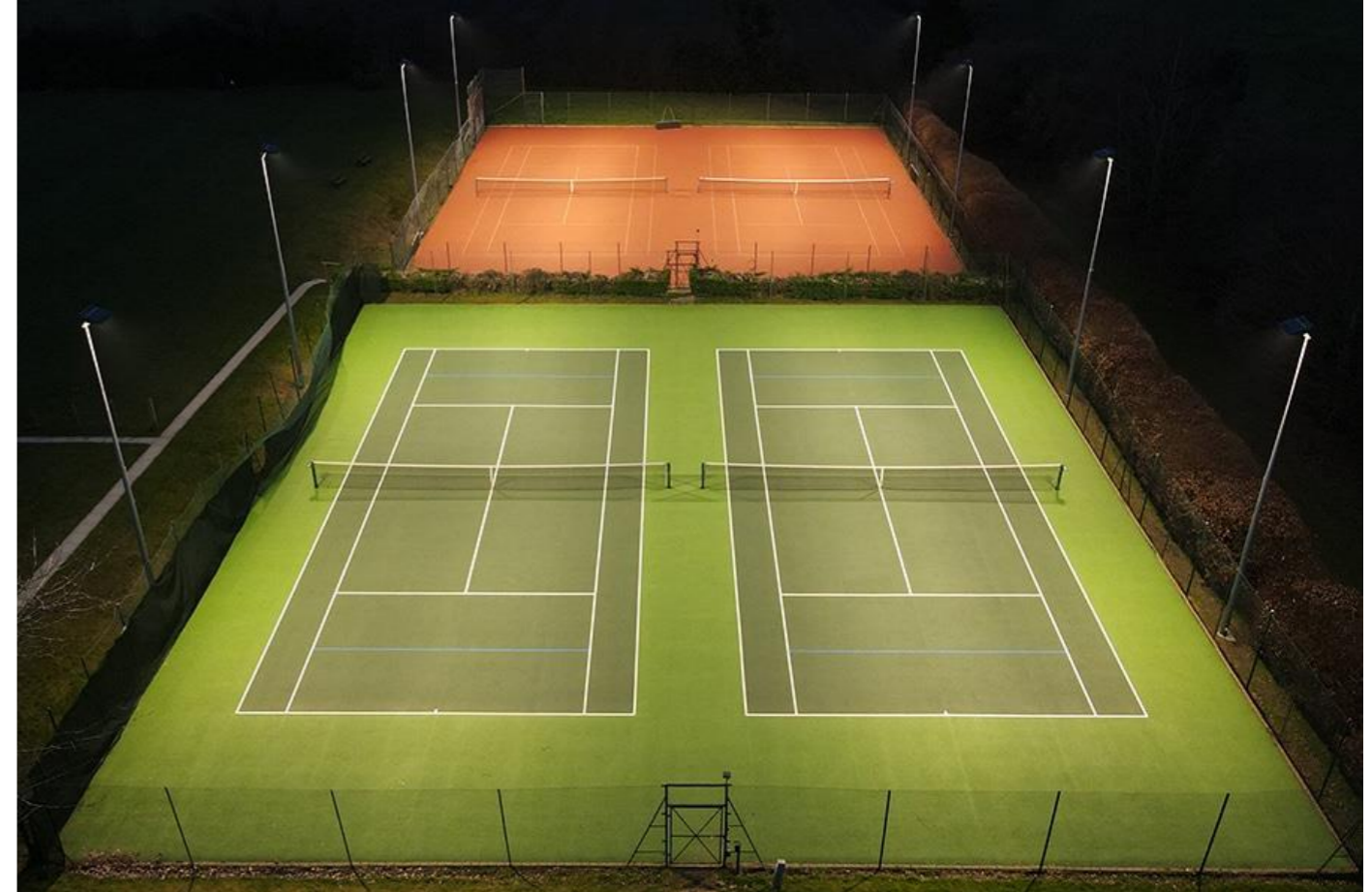
Column mounted floodlights – Illustrative Image.
