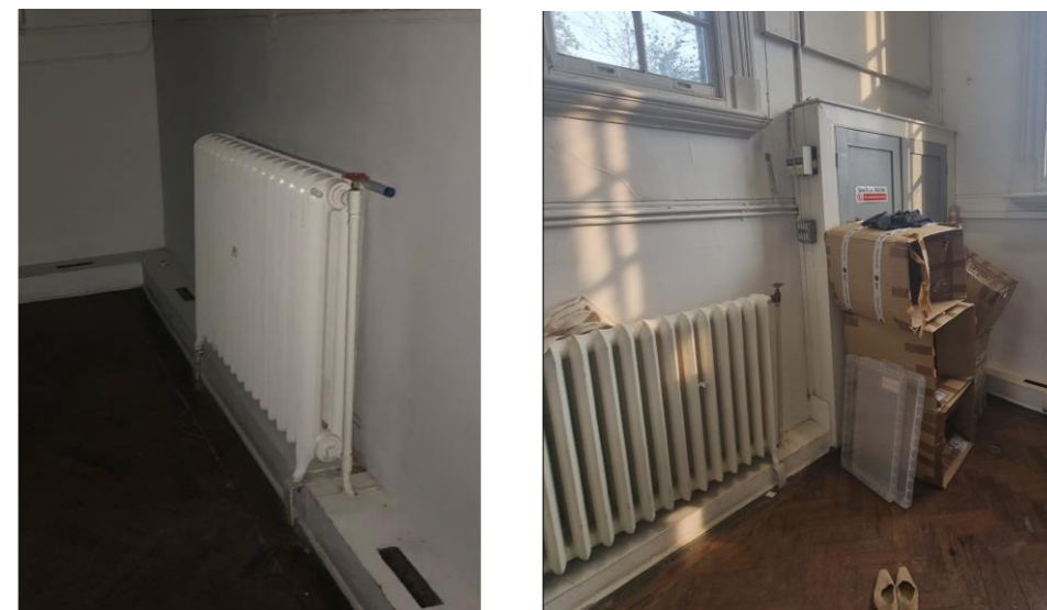
Fig 4. Existing services have been installed surface mounted with no consideration for the historic building fabric
