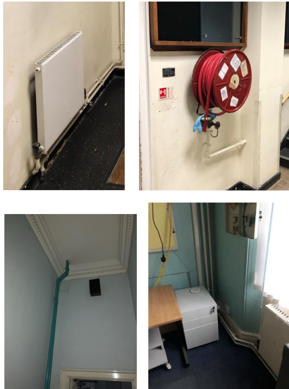
Fig 2. Existing services have been installed surface mounted with no consideration for the historic building fabric
