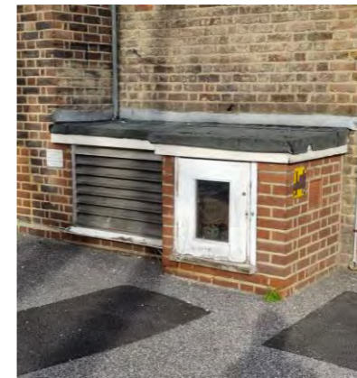
Meter house; Kneller Hall
