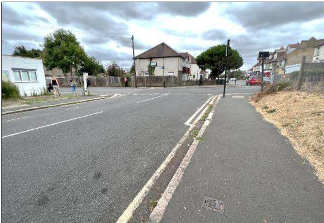
Figure 4.10 Lack of Crossing Facilities on Maswell Park Road / Hounslow Ave
