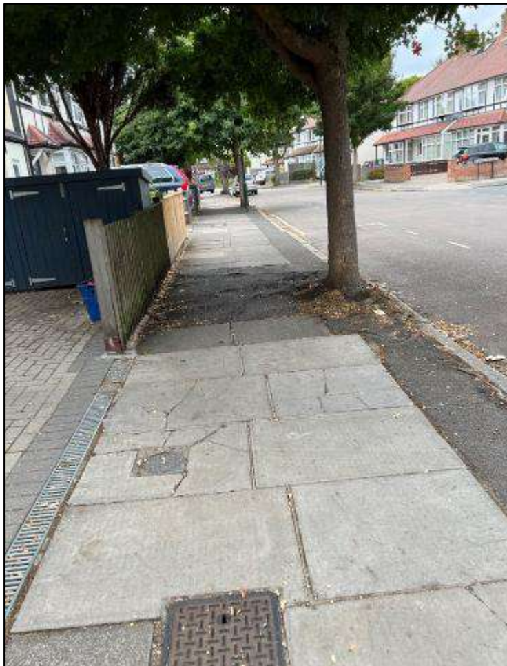
Figure 4.14: Damaged Footway on Chudleigh Road (Photograph 4F)
