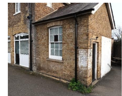
Photo 4 Failed Brick Arch above sash window at the rear storage room in the Guards House
