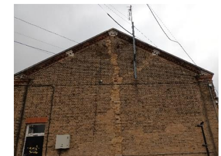
Photo 6 Significant vertical crack to the external gable wall at the rear of the Band Practice Hall
