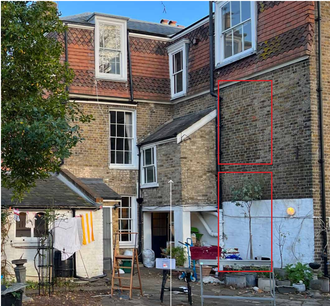
Existing Rear elevation - showing blocked in windows at ground and 1s floors
