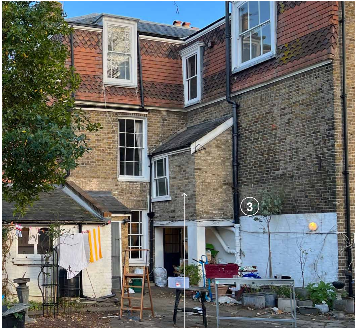
Existing Rear elevation - showing 1st Floor WC Extension (20th Century later addition to original building)
