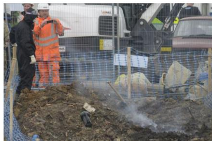
The scene at Blacksole Bridge after wartime explosives were found in the railway cutting
