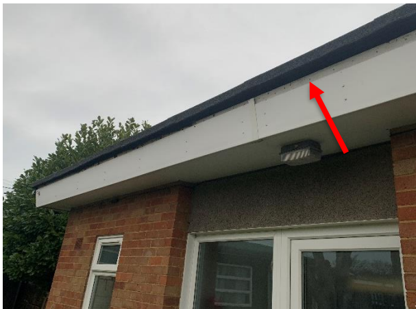
Plate 4.22 Lifted Roofing Felt (Western Aspect)
