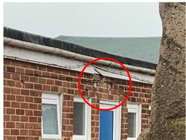
4.8: Damaged Brickwork (Northern Elevation)
