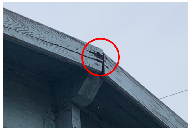
Plate 4.11: Damage to Wooden Roof Apex (Western Aspect)
