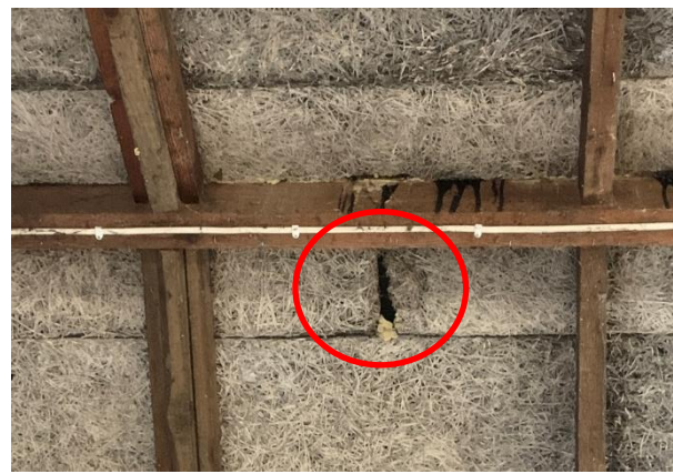
Plate 4.18: Gap in The Ceiling Insulation
