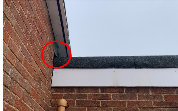
Plate 4.4: Lifted Roofing Felt (Western Aspect)
