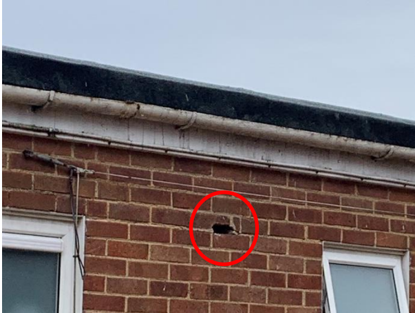
Plate 4.9: Hole in the Brickwork (Northern Elevation)
