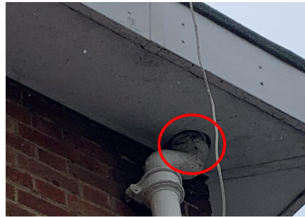
Plate 4.6: Gap in the Soffit (Eastern Elevation)
