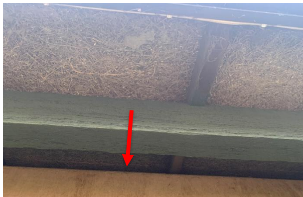
Plate 4.16: Gaps At The Eaves (Southern Aspect)
