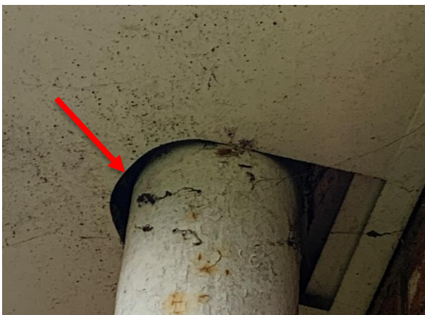
Plate 4.7: Gap in the Soffit (Eastern Elevation)
