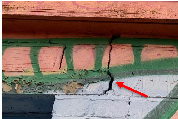
Plate 4.14: Damaged Brickwork (Eastern Aspect)
