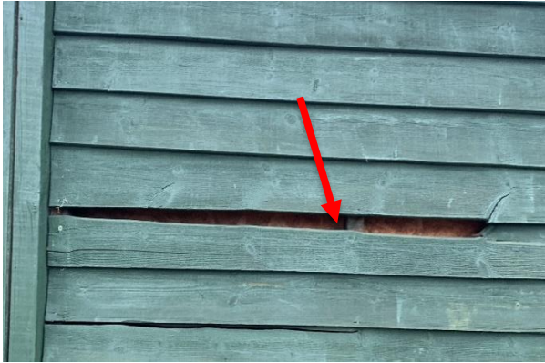
Plate 4.12: Missing Wooden Cladding (Southern Aspect)
