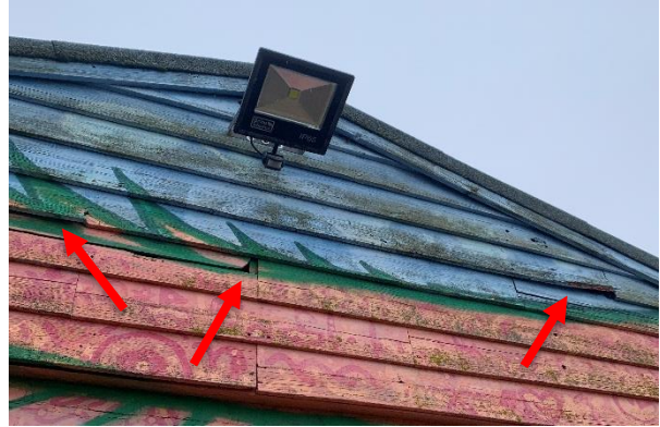
Plate 4.13: Damaged Wooden Cladding (Eastern Aspect)
