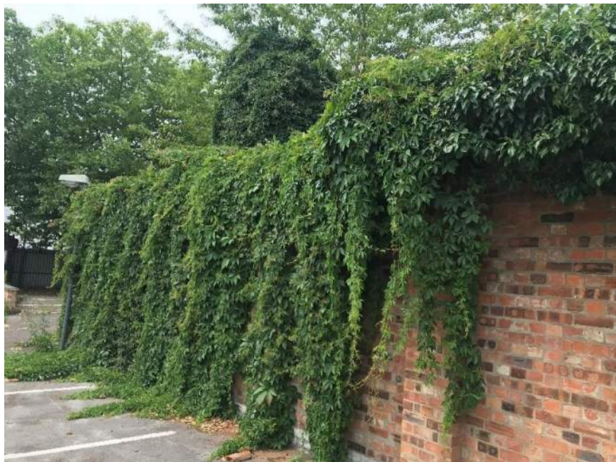
Plate 6 – Example of Virginia creeper overgrowing wall from neighbouring property within the north of the Site.
