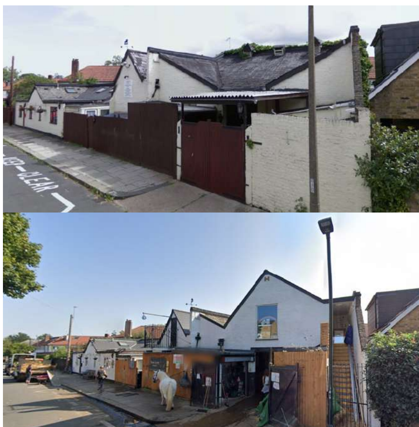
Building elements on the site in 2015 (top) and after works 2015/2016 (lower). “Undesigned” new and old roofs to buildings at the south of the site are used to highlight heritage quality in the council’s draft BTM assessment.
