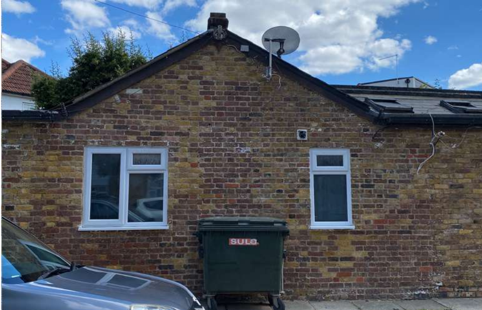
Mixed brickwork on the front elevation gable evidencing rebuild, repair, and with the later brickwork of the flat roofed extension distinct (RHS of photo - and generally in London yellow stock brick). The applicant notes in particular the yellow stock brick below the apex of the gable in the above photograph with a red brick generally below, and that there is little visibly apparent trace of the former window to the gable that is shown in the above-page 1960s photograph.
