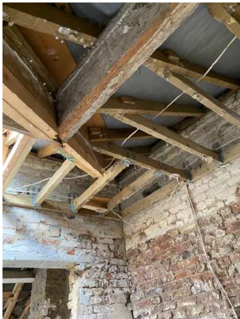
Old purlins supporting the pitched roof rafters have been retained through the re-roofing construction.
