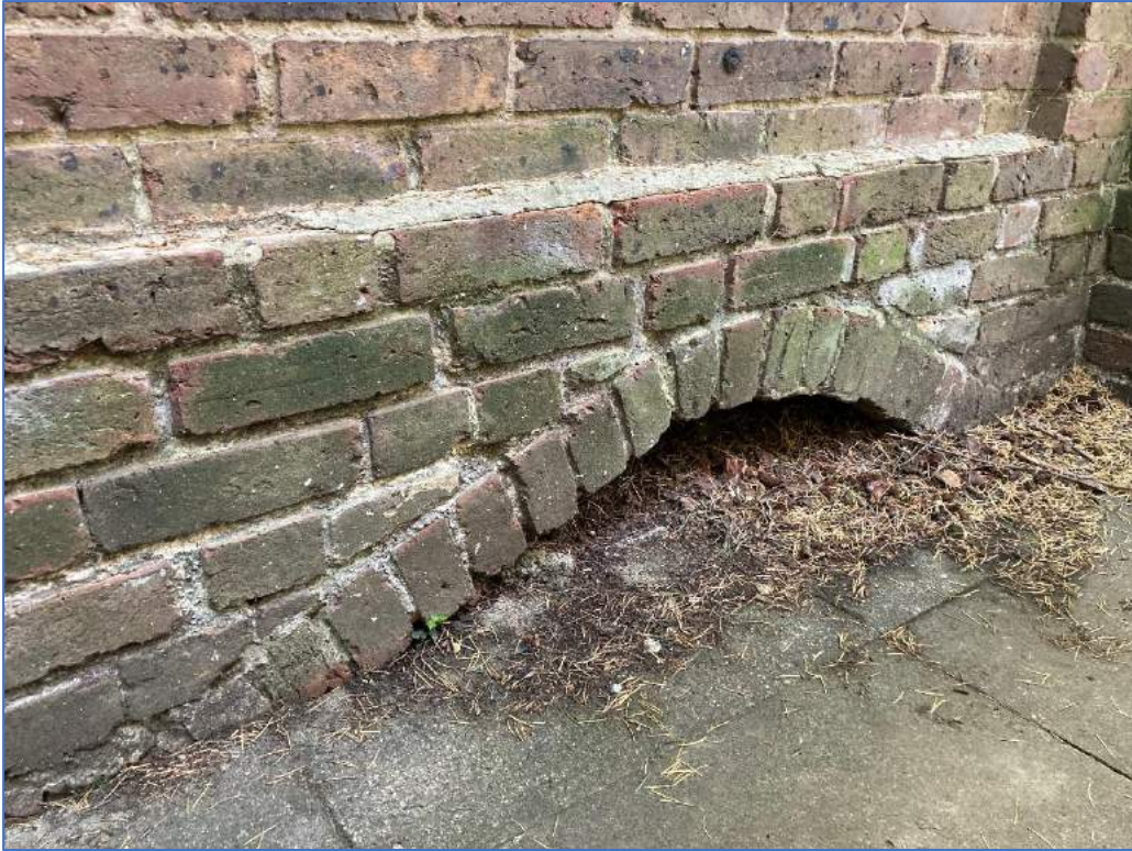
Plate 11: South-facing detail of archway at the base of the 19 th century boundary wall along the east boundary of the Site
