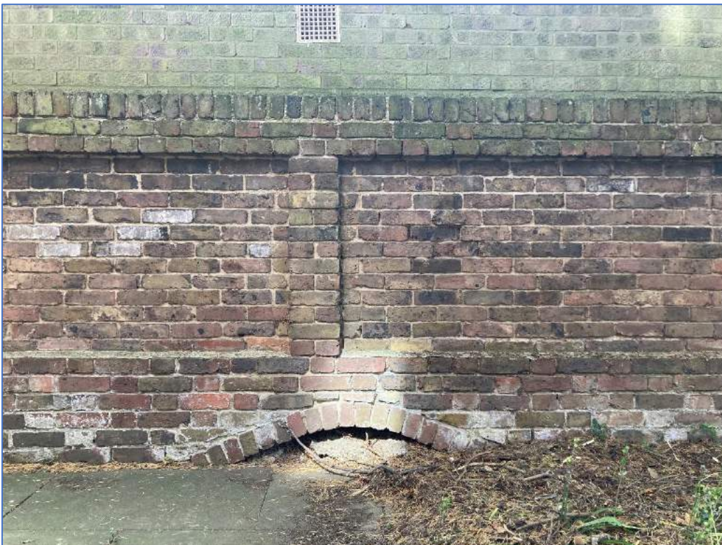
Plate 12: Southeast-facing detail of archway at the base of the 19 th century boundary wall along the east boundary of the Site
