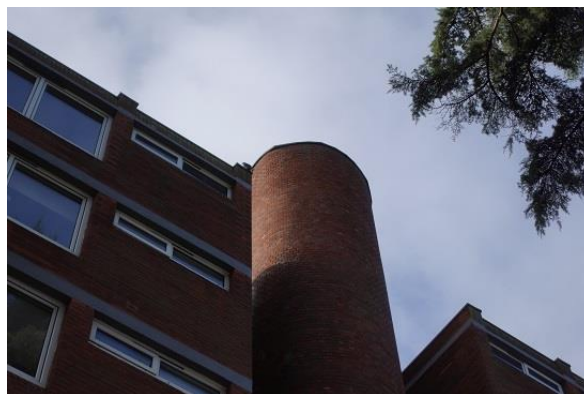
Plate 4.4: Lifted Lead Flashing on the Lift Tower
