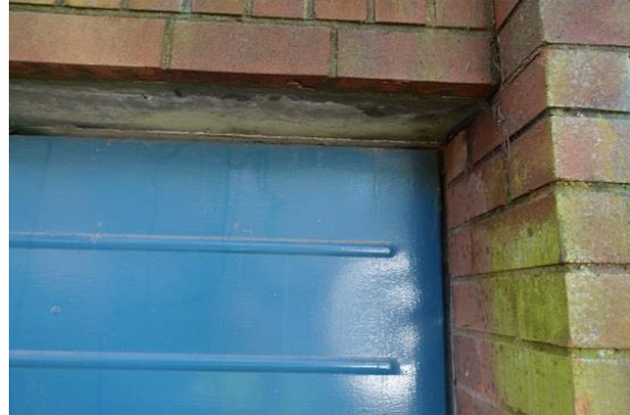
4.7 Gaps Between Doors and Brickwork
