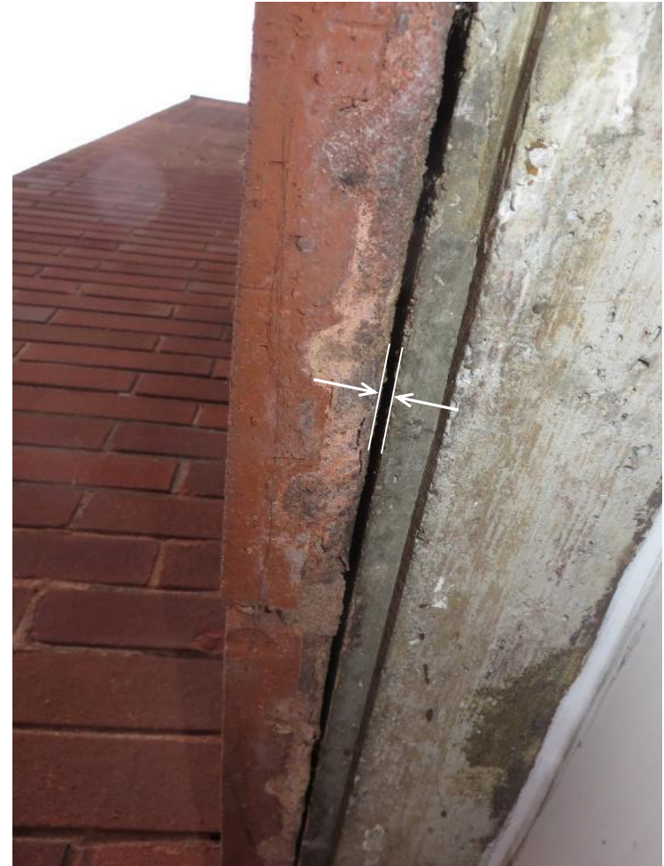
Visible gap between the concrete lintel and the vertical bedding mortar.
