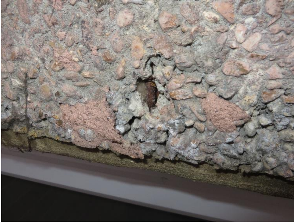
First floor rear elevation. Typical surface honeycombing, corroding reinforcement visible.
