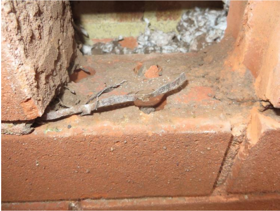
Three courses above the brick slips. Expanded metal mesh within the horizontal brickwork joint.
