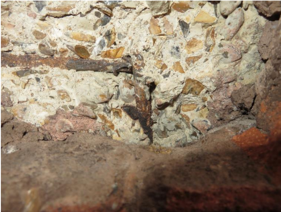
The reinforcement had surface corrosion.
