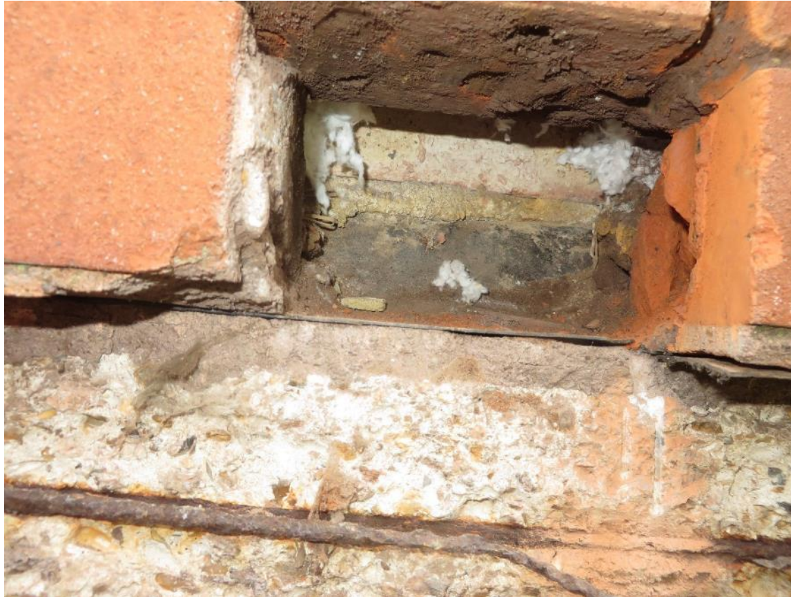
Cavity tray bituminous sheet. Cavity tray height only 50mm. Joints in inner and outer leaf's don't align vertically. Cavity tray covered in mortar and construction debris. Blown fibre insulation within cavity.
