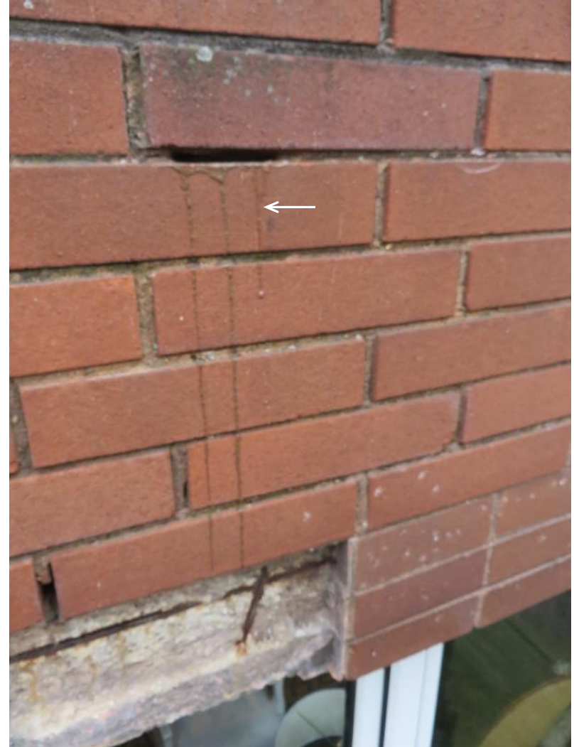
During an investigation into the wall ties on the third floor rear elevation. Water seeped out of the horizontal mortar joint, when it was disturbed.
