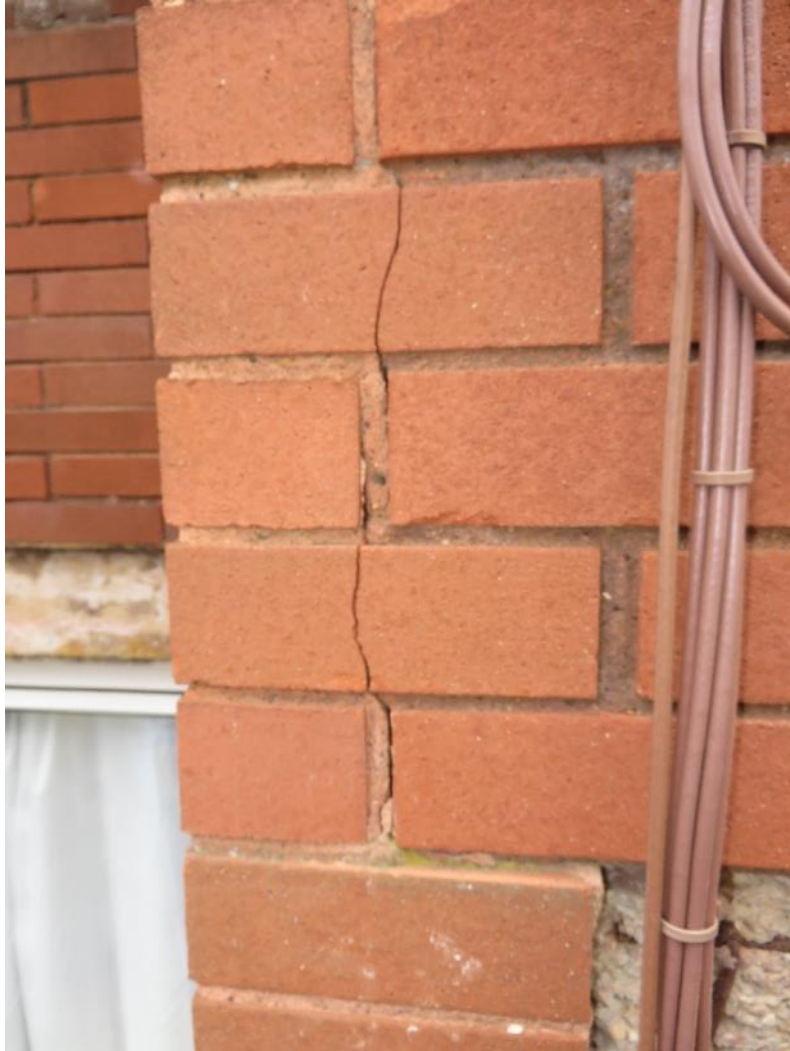
Vertical cracking in the brickwork above a lintel.
