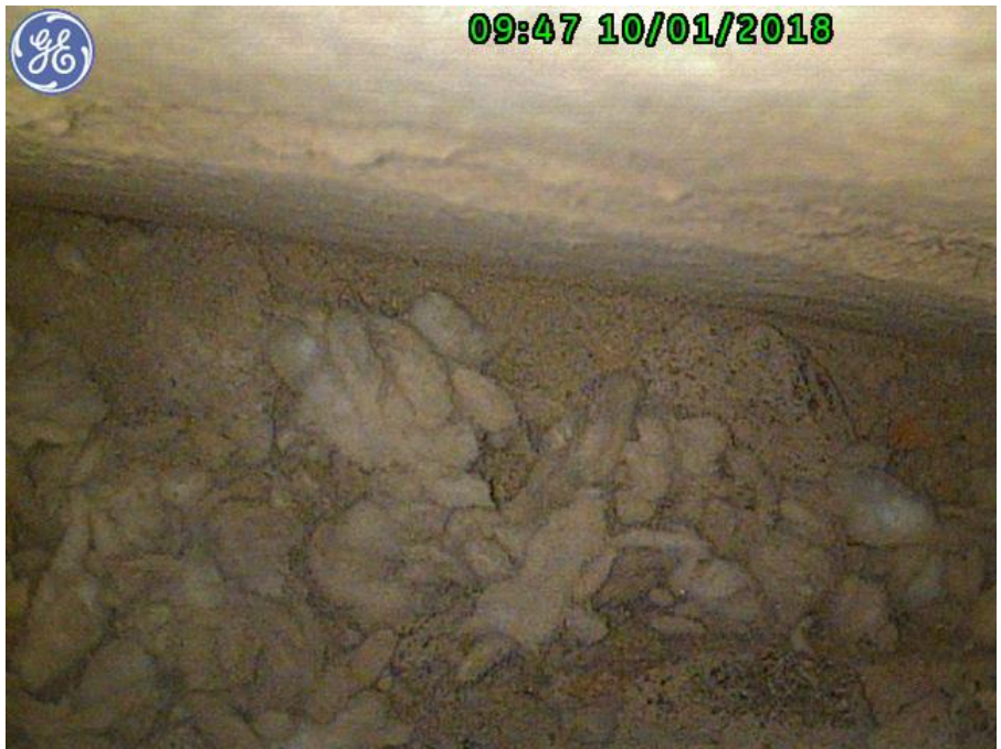
Detail of the debris sitting on the cavity tray.
