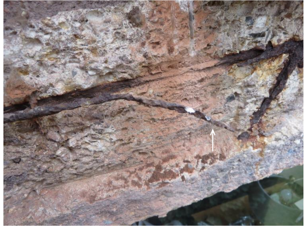
Third floor rear elevation. One hundred percent loss of section to the horizontal top reinforcement.
