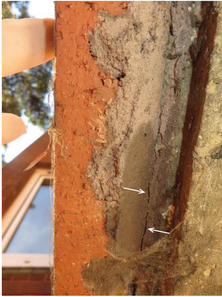
Crack between the concrete lintel and the vertical bedding mortar.
