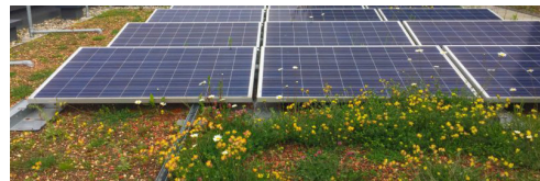
Fig. 3 & 4 PV Panels mounted on green flat roof
