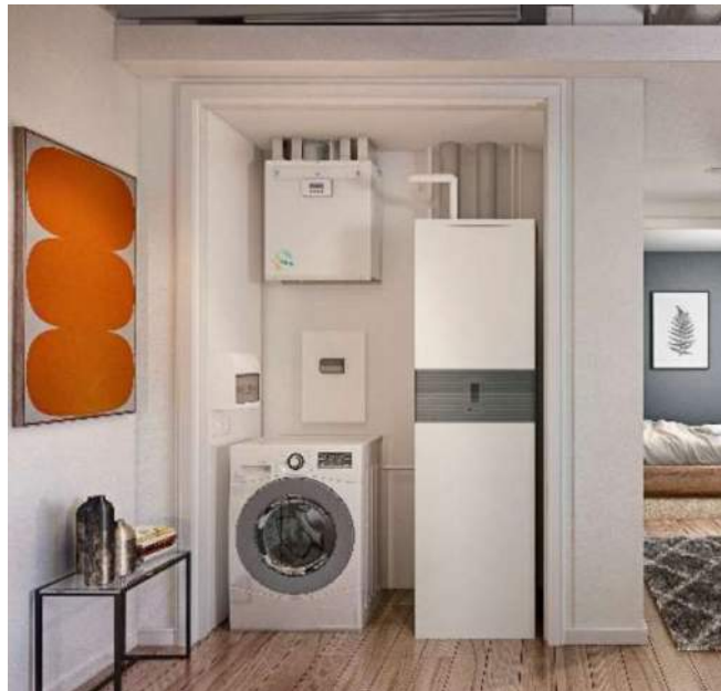
Figure 2 – A heat pump and hot water cylinder within an apartment utility cupboard
