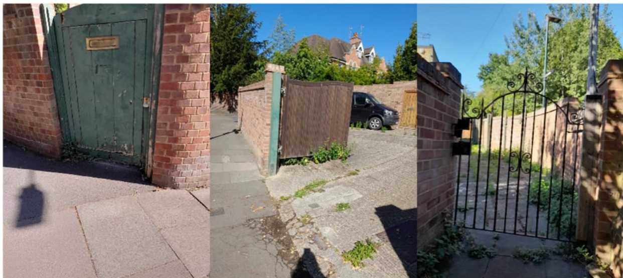
Figure 5-1 Gaps in existing site perimeter wall
