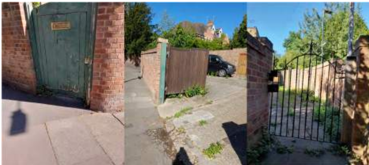
Figure 5-1 Gaps in existing site perimeter wall
