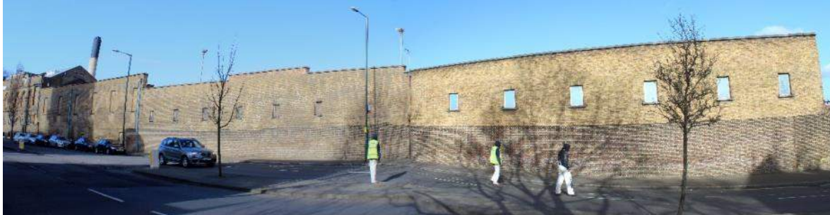
Plate 28 External elevation of south boundary wall with section 1 (left end) and section 2 (right end) (2017)
