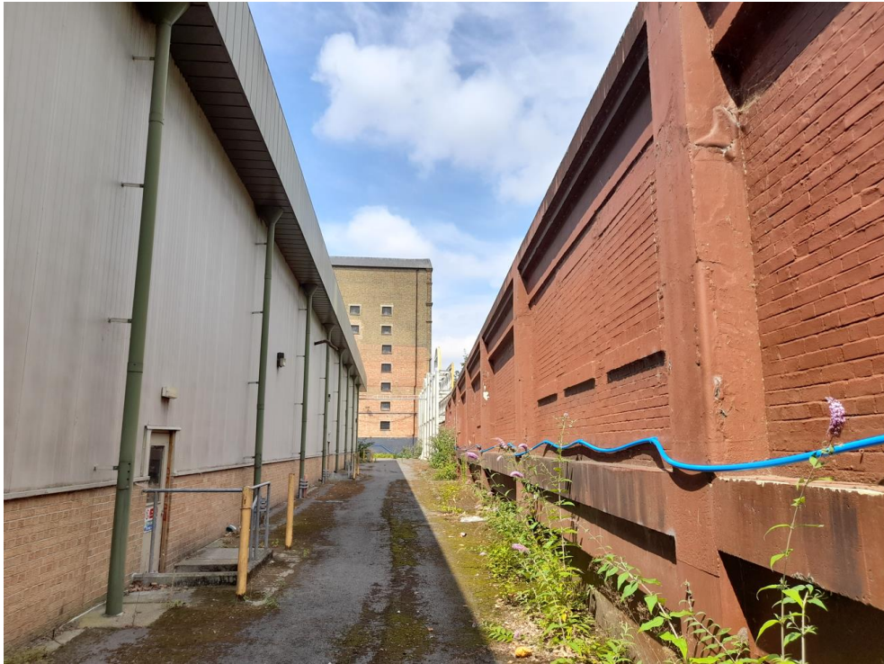
Plate 10: Section of northern boundary wall (HA004) adjacent to the maltings building (HA003), viewed from within the site. Existing view to west.
