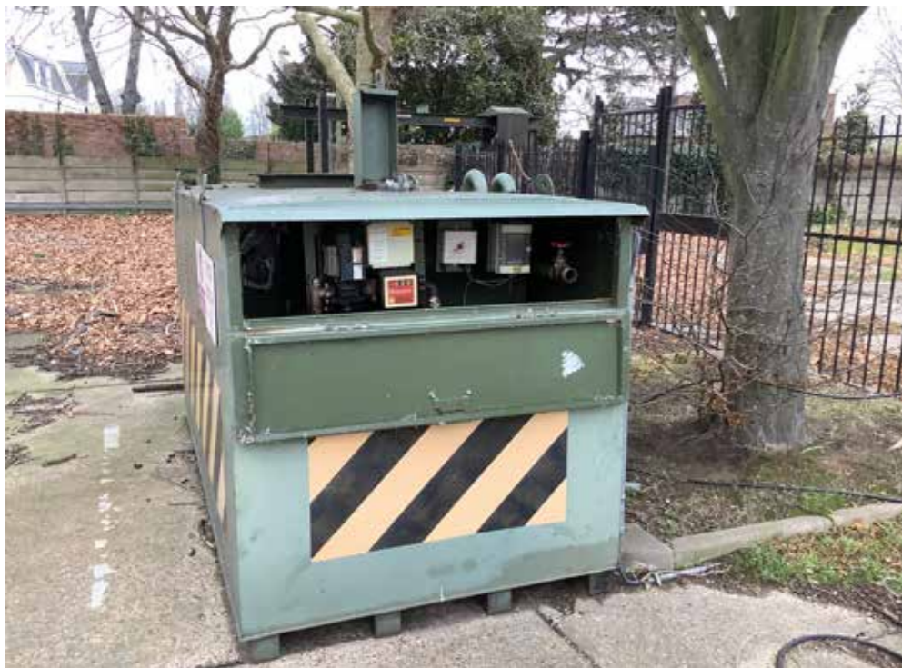
Portable diesel tank at north boundary of brewery West Site
