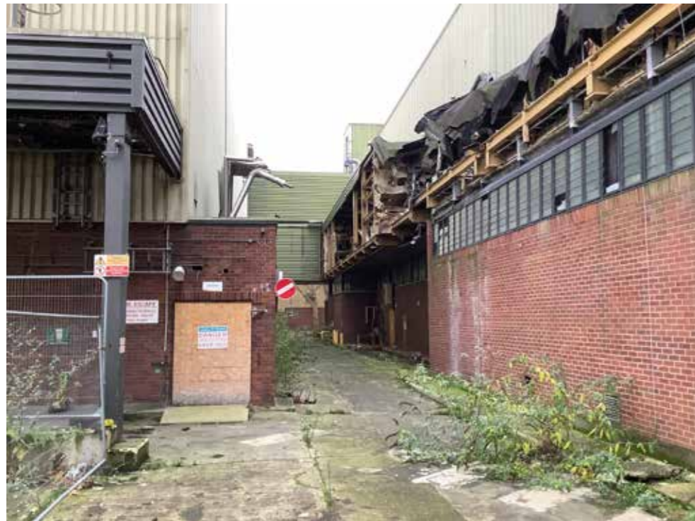
Partial demolition of West Site brewery structures as part of tank removal
