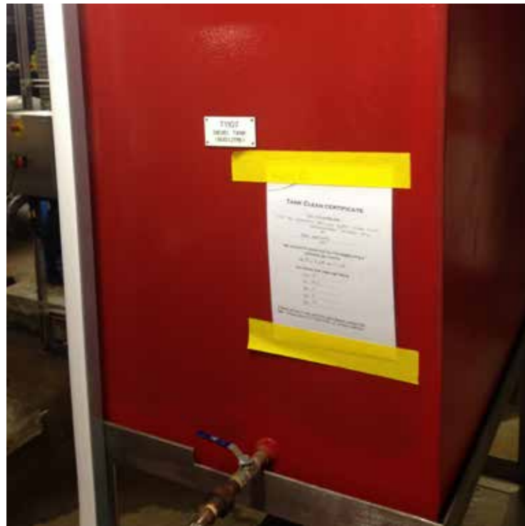
Decommissioned diesel tank in Production Office basement
