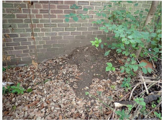
Photo 8 Former badger sett on garage wall.
