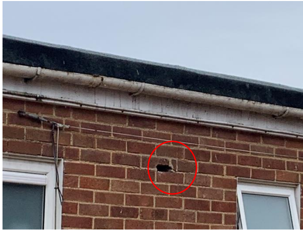
Plate 4.9: Hole in the Brickwork (Northern Elevation/Southern Edge of Courtyard)
