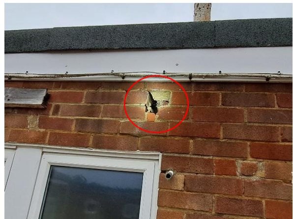
4.8: Damaged Brickwork (Northern Elevation/Southern Edge of Courtyard)
