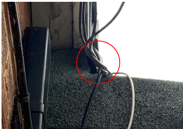
Plate 4.5: Lifted Roof Felt (Eastern Elevation)
