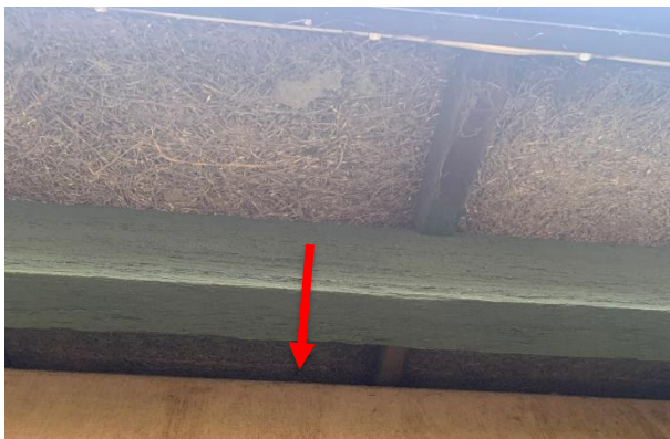
Plate 4.16: Gaps At The Eaves (Southern Aspect)
