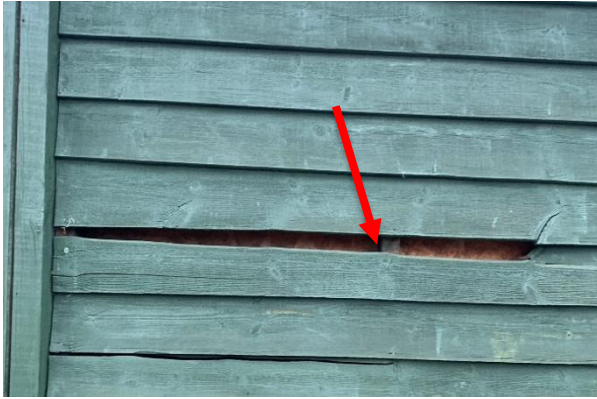
Plate 4.12: Missing Wooden Cladding (Southern Aspect)
