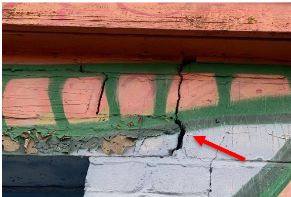
Plate 4.14: Damaged Brickwork (Eastern Aspect)
