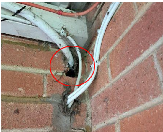
Plate 4.7: Gap in the brickwork (Southern Elevation)
