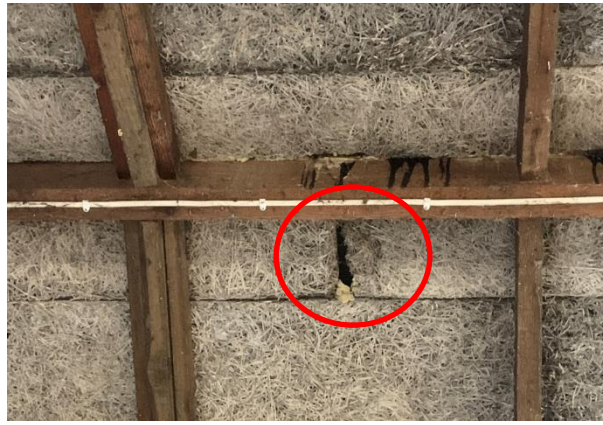
Plate 4.18: Gap in The Ceiling Insulation
