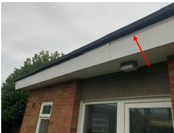
Plate 4.22 Lifted Roofing Felt (Western Aspect)
