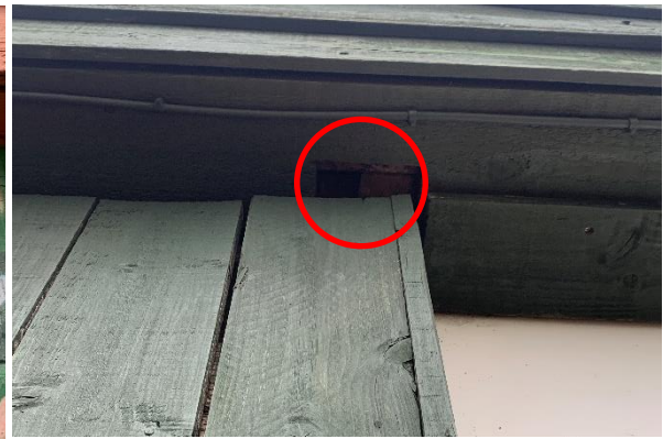
Plate 4.15: Loose Fitting Joins (Southern Aspect)
