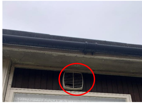
4.20: Damaged Roof Vent (Northern Aspect)
