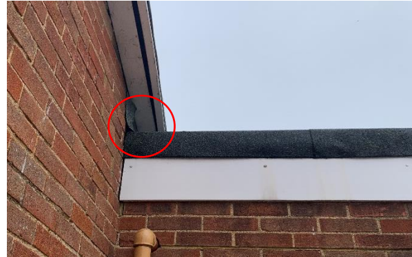
Plate 4.4: Lifted Roofing Felt (Western Aspect)
