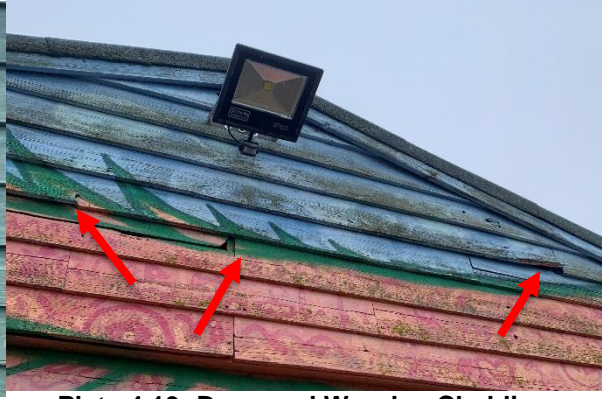
Plate 4.13: Damaged Wooden Cladding (Eastern Aspect)
