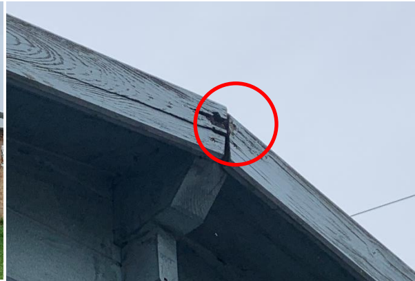
Plate 4.11: Damage to Wooden Roof Apex (Western Aspect)
