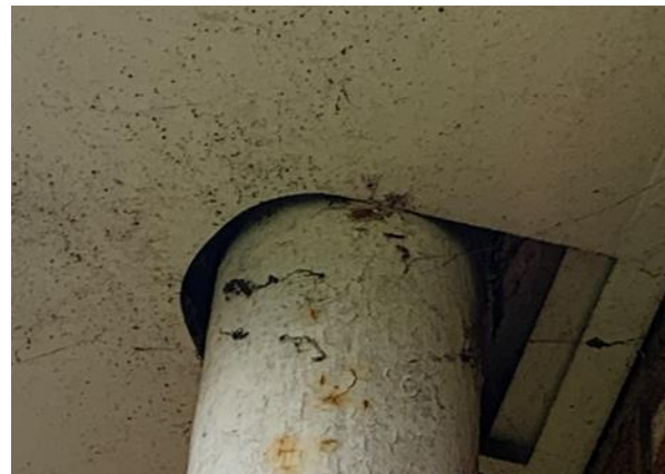
Plate 4.6: Gap in the Soffit (Eastern Elevation)
