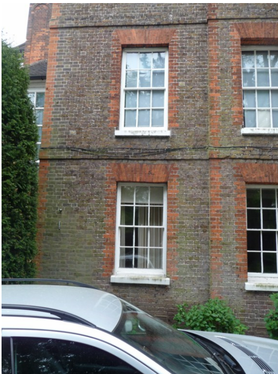
Slight distortion of spandrel panel on west elevation
