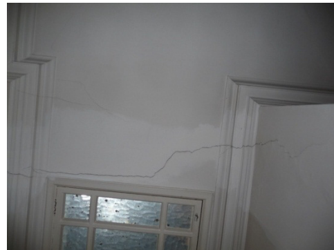
Cracking in ceiling
