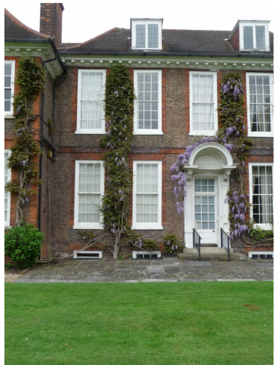
Slight drooping of pier between windows
