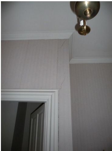
Cracking in partition wall
