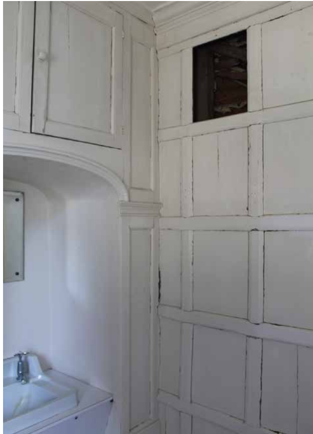
3.16 Square panelling in toilet in north east corner of the entrance hall (G5)
