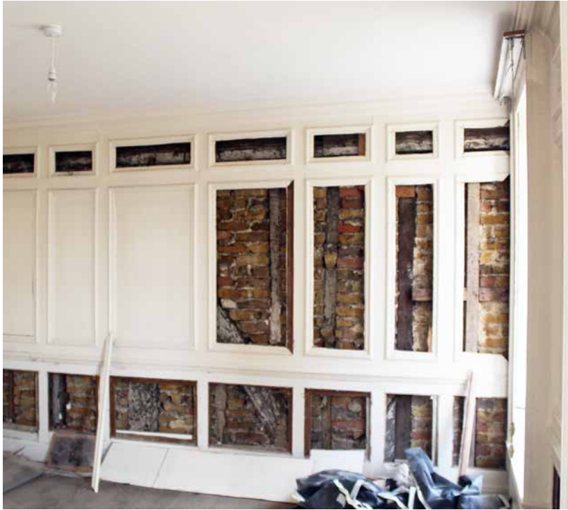
3.21 The first floor north west room (F2) showing timber framing in south wall
