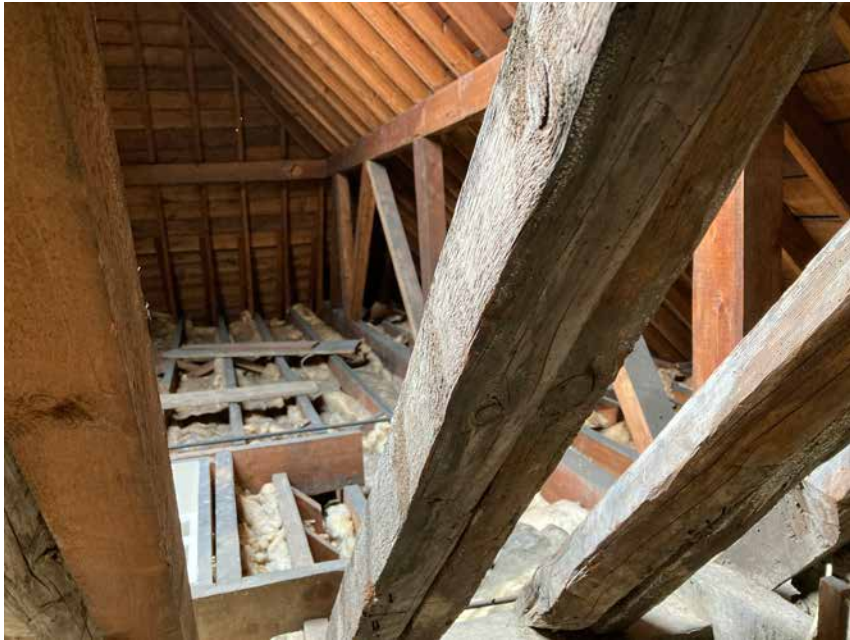
5.3 Rafters on the south side of the 18C roof, looking into the roof of the south Edwardian extension
