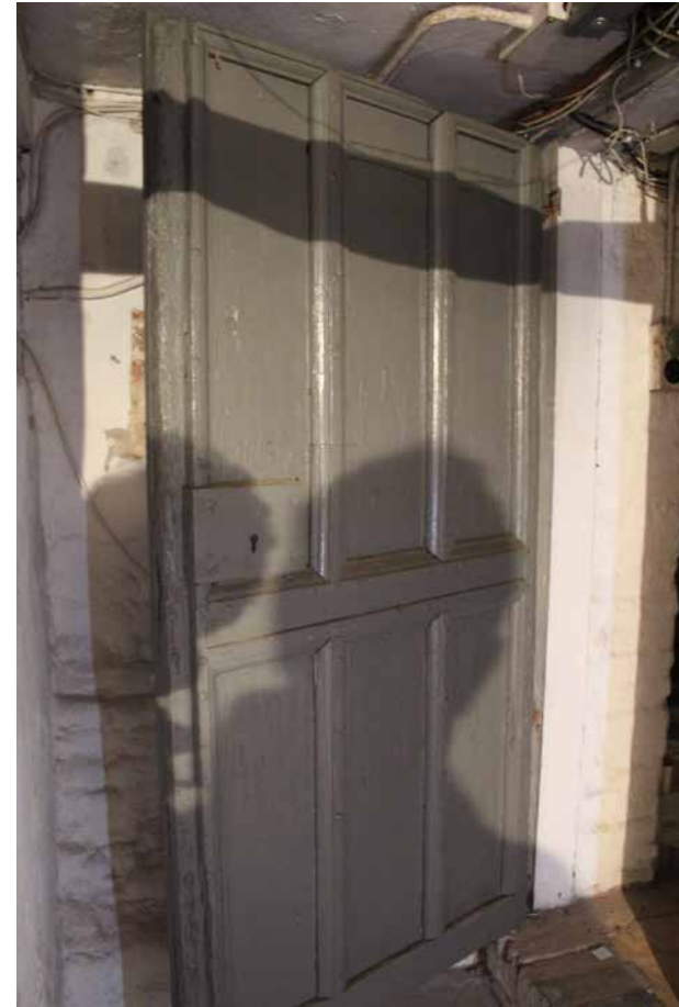
3.12 Possibly late 17C-early 18C door in the basement (at the south end of B4 leading to B3)
