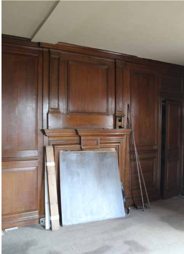
3.30 The 'oak' panelled room in the southwest corner at first floor level (F1)
