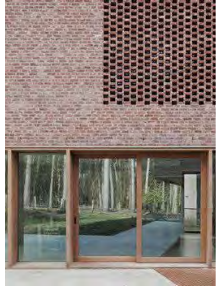
Perforated brickwork to protect views to and from the internal spaces, with deep set glazing below.
