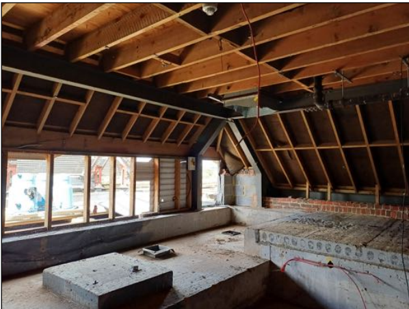
Image 12: There is a void space in the main section of the building which has an open side with mesh covering.
