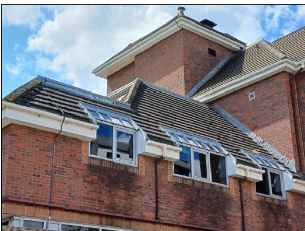
Image 8: The roof tiles present are large concrete tiles with no lifting and the soffit boxes are in good condition with no gaps.
