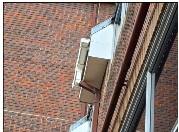
Image 9: Lead flashing is present around the flat roof of the extension. It is mostly flat but there are some gaps around the metal window frame though this is unsuitable for roosting.
