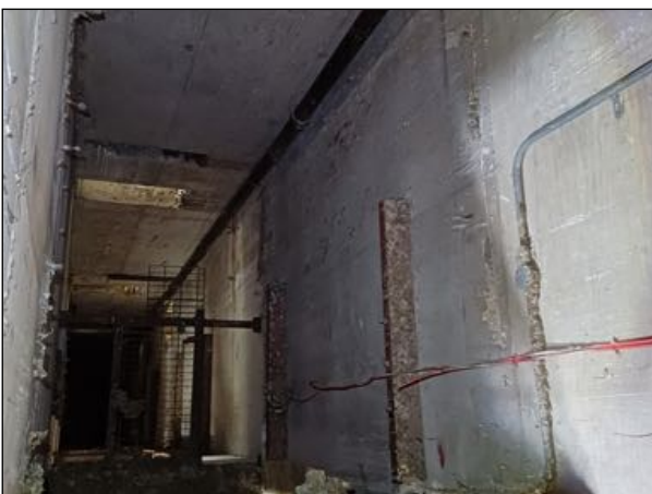
Image 14: One of the lift shafts present is open from the top floor void space but has no roosting opportunities.
