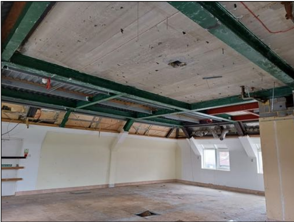
Image 10: A view of the second floor of the extension. There is no void present in the extension.
