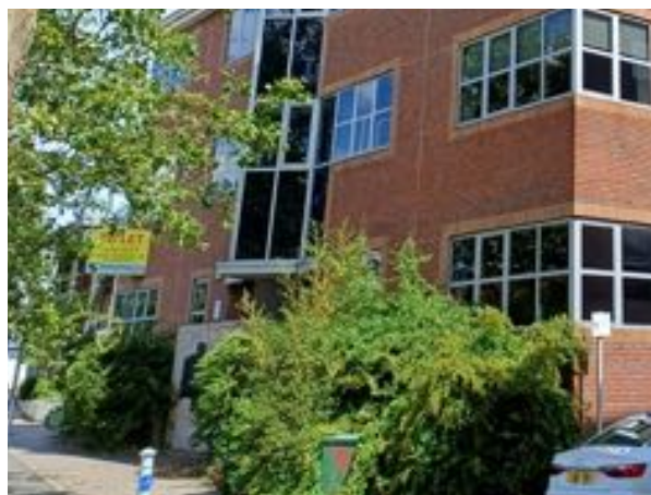
Image 3: Overgrown ornamental planting at the front of the building.
