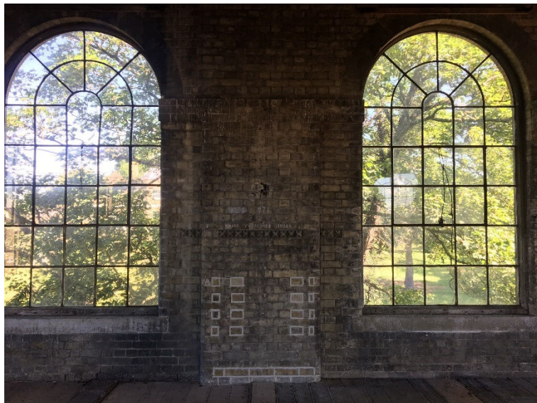
Location: Karslake – Former Bean Engine House Description: General view of interior brick work detailing
