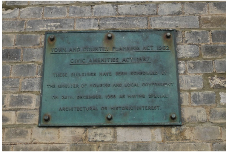
Figure 13 – Metalwork – Discolored signs or features
