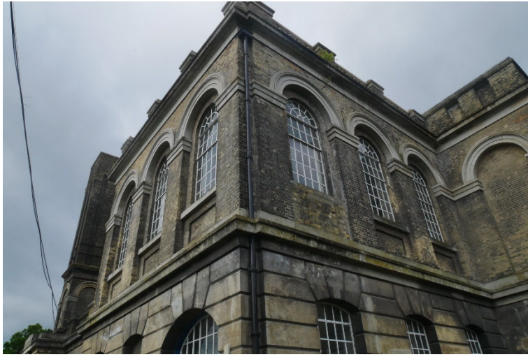
Figure 11 – Metalwork – defective rainwater goods
