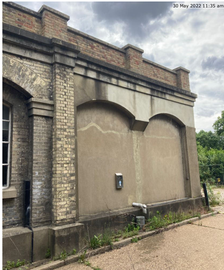
Figure 9 – Render, plaster defected finish
