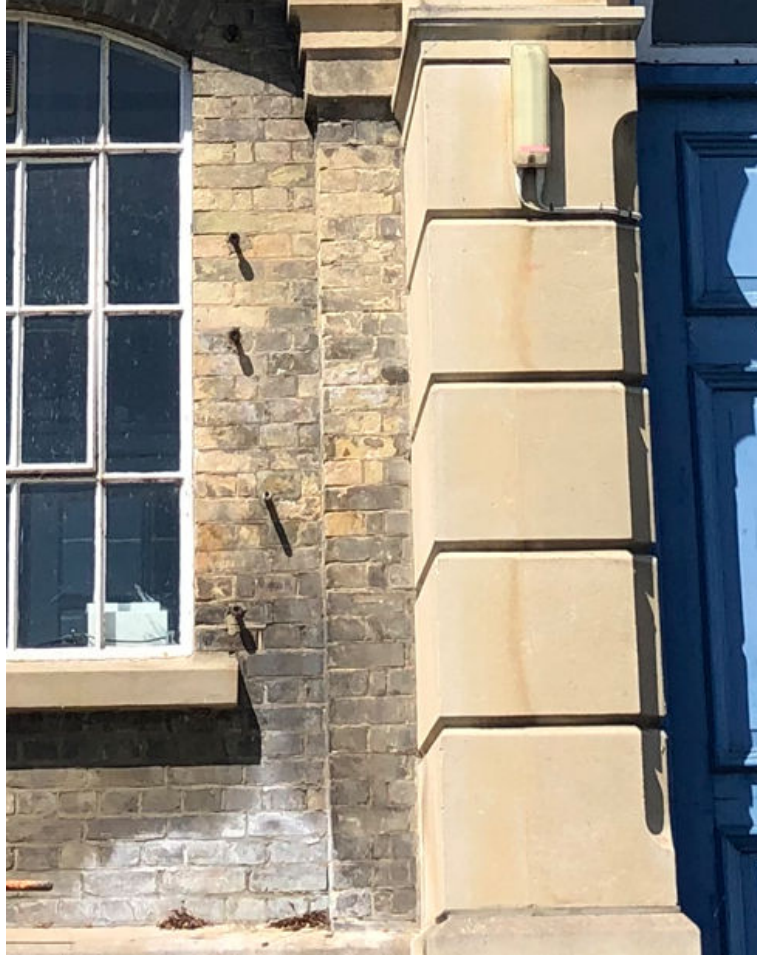
Figure 1 – Brickwork – discolouring and staining
