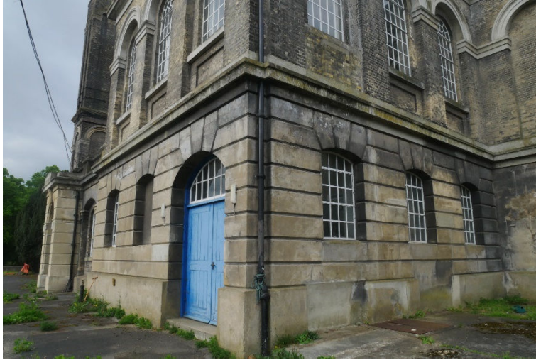
Figure 6 – Stonework, render, plaster – discolouring and staining
