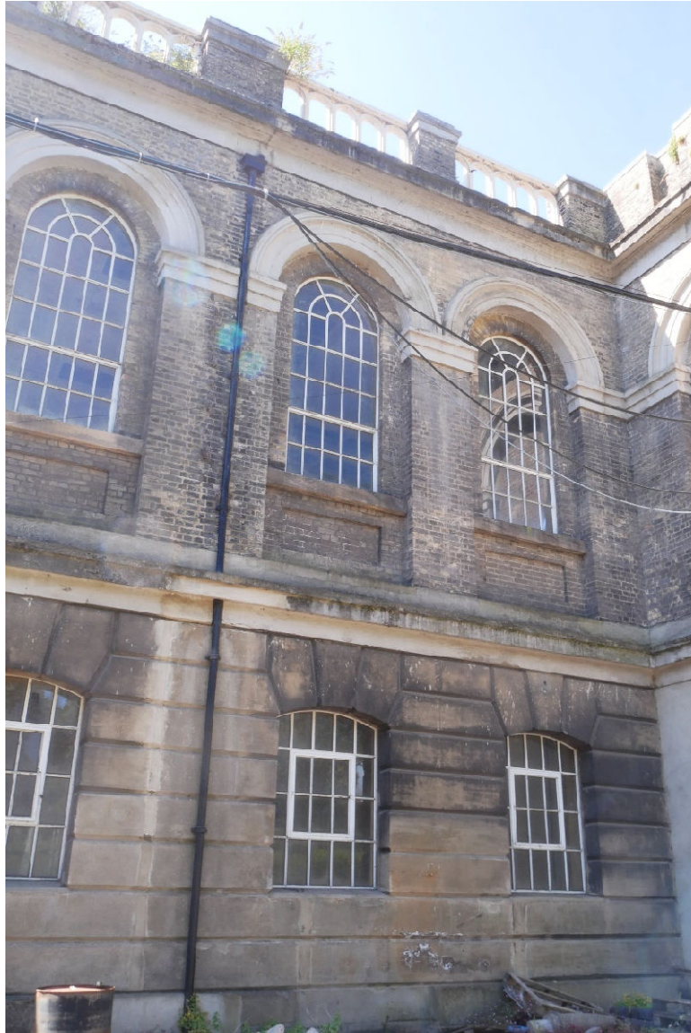
Figure 1 – Brickwork – discolouring and staining
