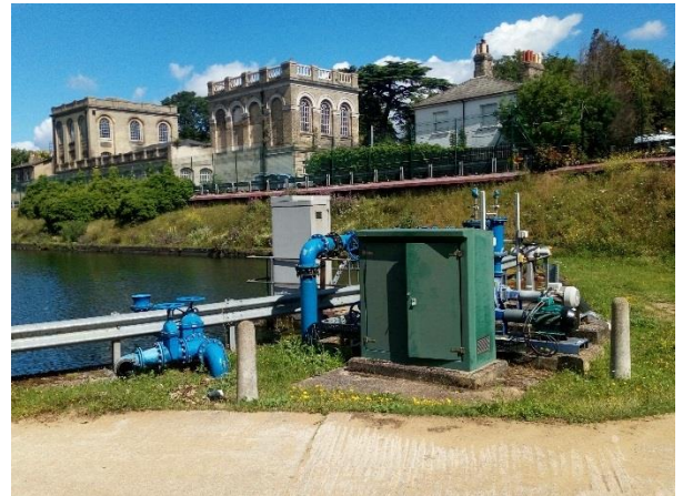
Figure 2.4: taken from the operational waterworks towards the site, showing the southern edge of the site in the background.
