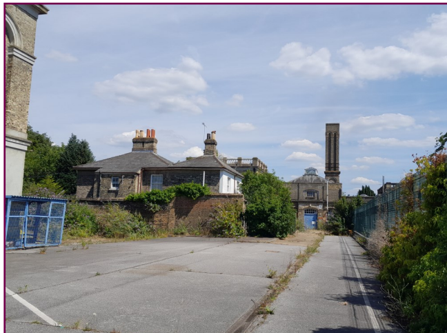
Photograph 6: Vegetation growing through hardstanding
