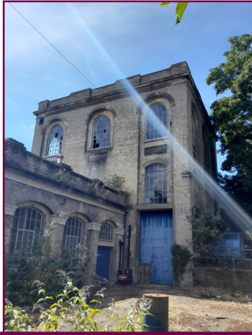
Photograph 1: TN1—B9 broken glass on top floor (north side)
