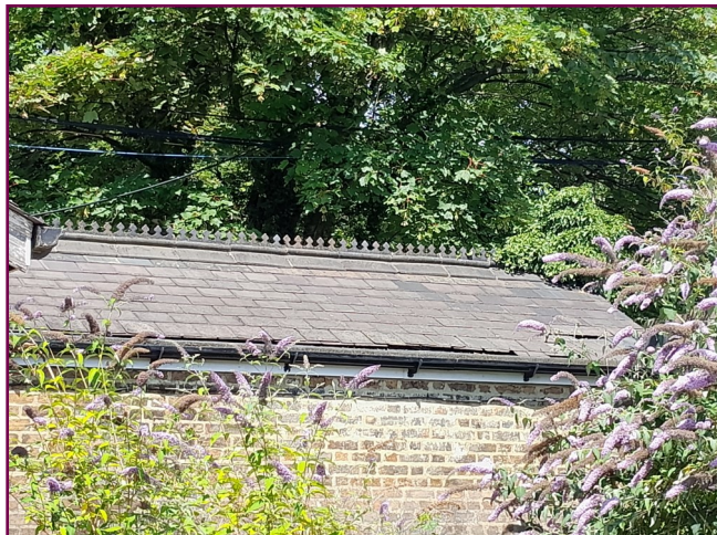
Photograph 4: TN3—missing roof tiles
