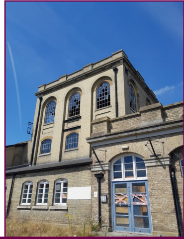
Photograph 2: TN1—B9 broken glass on top floor (south side)
