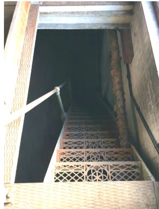
Figure 59: Steel staircase with decorative perforated treads leading up to The Beam's mezzanine level
