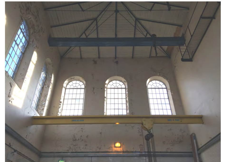
Figure 34: The interior of Ruston Building's two-storey engine house with round-headed non-original steel windows
