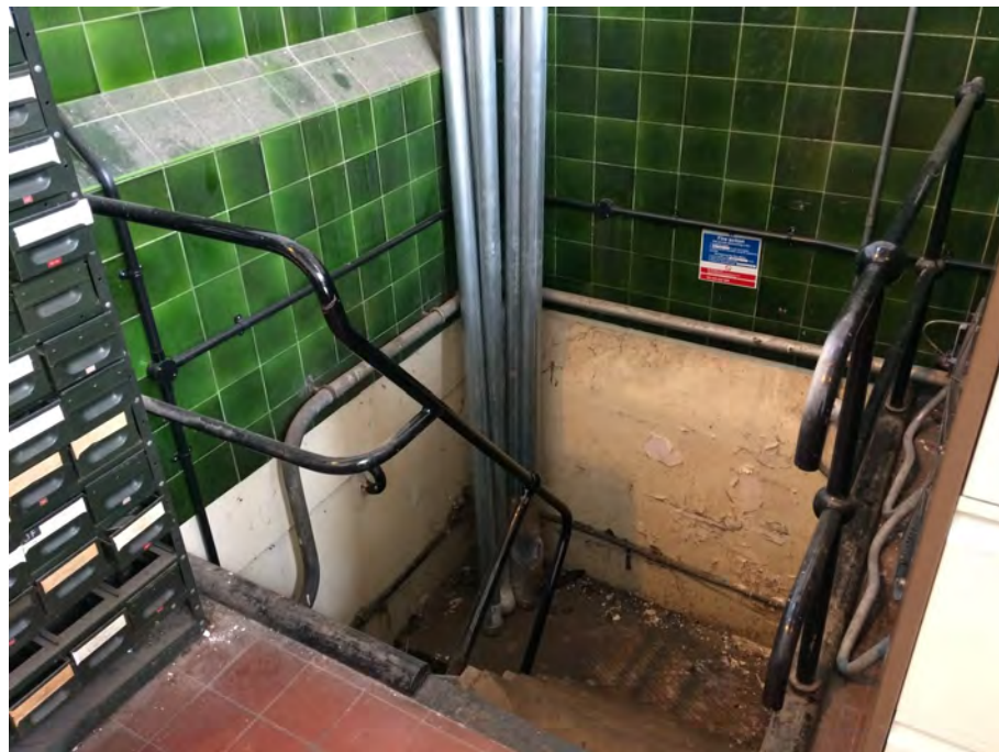
Figure 38: The staircase leading down to the basement under Ruston Building's engine house
