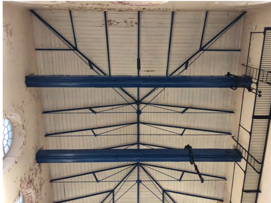
Figure 35: The roof structure of Ruston Building's engine house consists of composite wrought iron trusses with timber sarking boards and slate roofing
