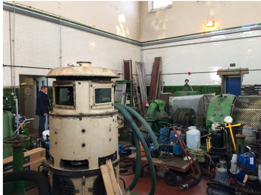
Figure 36: The interior of Ruston Building's engine house with Victorian white and green wall tiles
