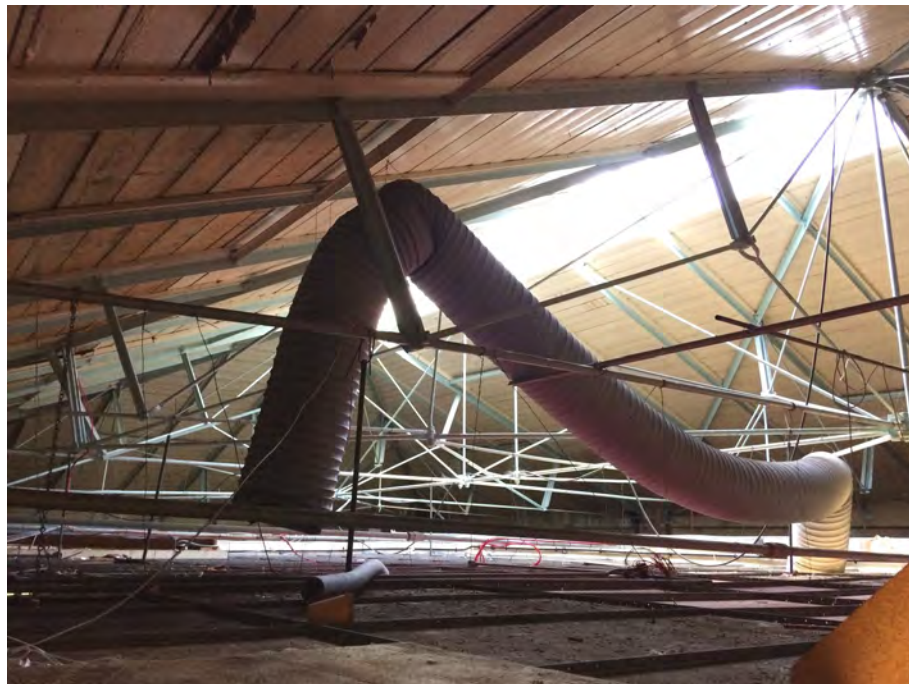
Figure 32: The roof structure of Ruston Building's boiler house consists of composite wrought iron trusses with timber sarking boards and slate roofing. A glass lantern sits along the ridge.
