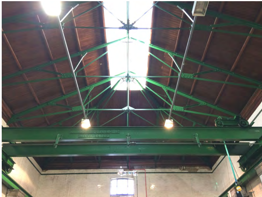
Figure 44: The roof structure of Ruston Building's southern block consists of steel trusses with polished timber sarking boards. A glass lantern sits along the ridge and steel gantry crane by The Vaughan Crane Co Ltd of Manchester is fixed below the roof structure.
