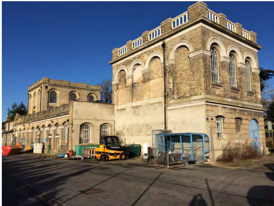
Figure 50: The rear of Karslake Building's eastern engine house where another late-nineteenth engine house once stood
