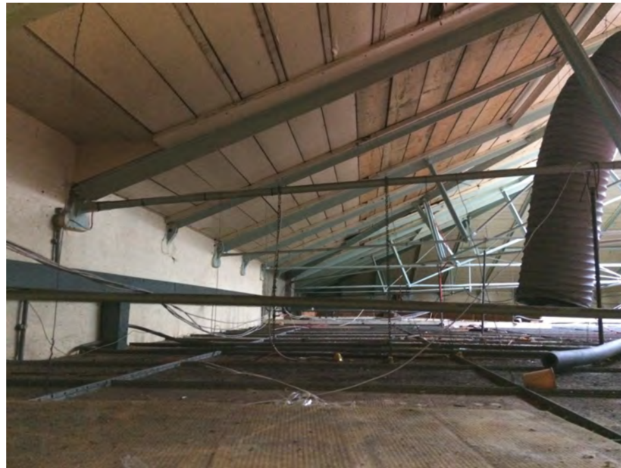
Figure 33: The roof structure of Ruston Building's boiler house consists of composite wrought iron trusses with timber sarking boards and slate roofing
