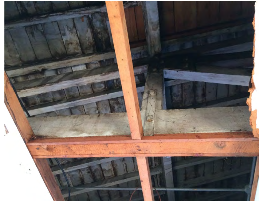
Figure 66: Timber and steel truss roof of the lean-to at the rear of The Beam
