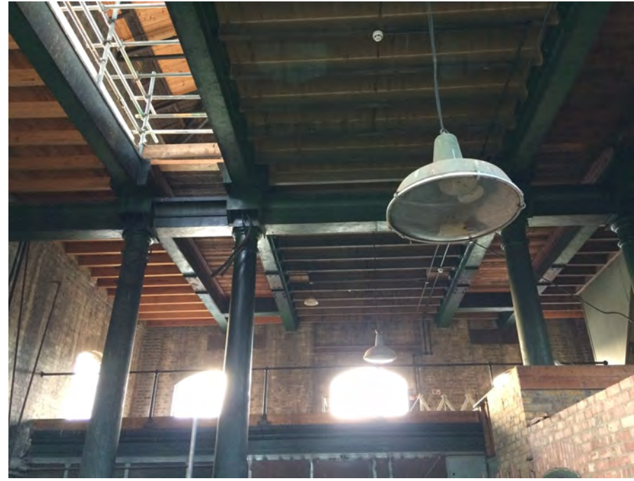
Figure 54: The steel structure holding up the second floor of Karslake Building's 'The Beam'
