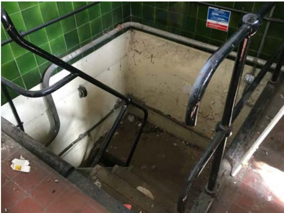
Plate 12: 2019 View showing access to existing basement in north east corner of Ruston & Ward building
