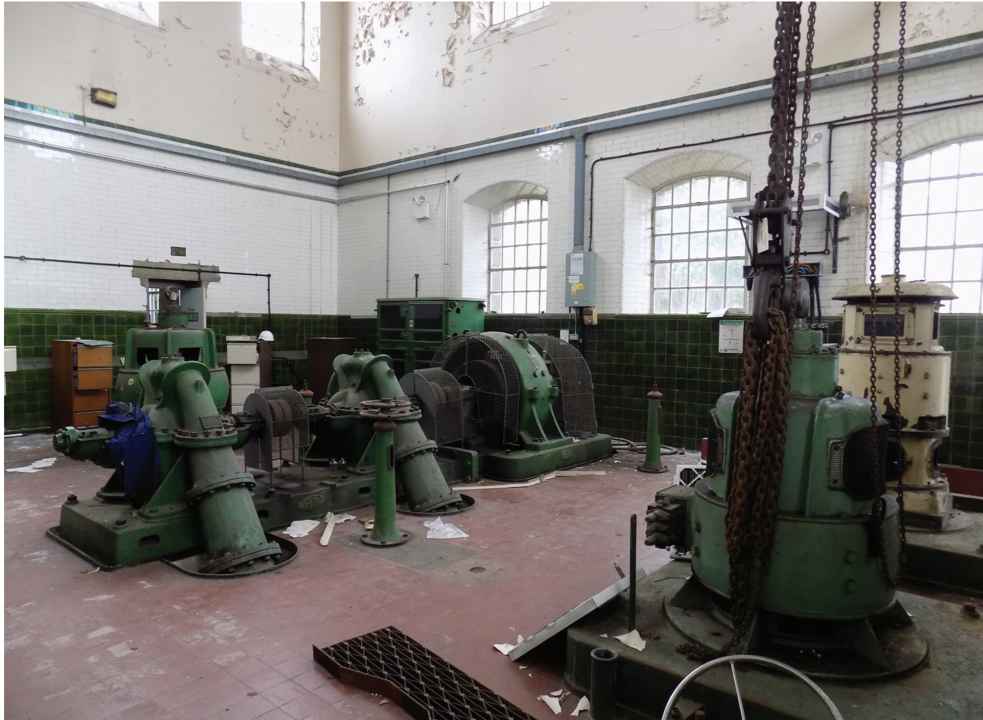
Figure 1: Ruston Ward former Bull engine house with electric pumps installed ca. 1936, with associated flooring and ceramic wall tiles. (Low-medium-significance). It is considered that the machinery has a low-medium level of interest and would tolerate relocation and preservation ex situ for interpretation purposes.
