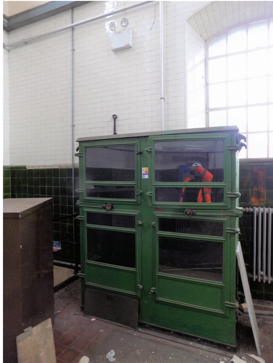
Figure 6: Double Leaf control cabinet for 1932 Harland electric centrifugal pumps, Ruston & Ward Engine House (low to medium significance)
