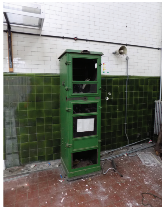
Figure 11: One of three 1932 Harland control cabinets for 1932 electric centrifugal pumps, Ruston & Ward Engine House (low to medium significance)
