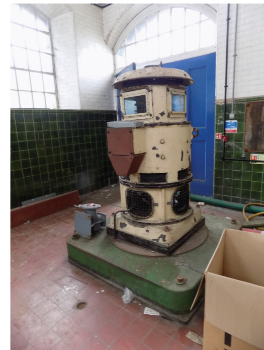
Figure 10: Replacement W H Allen DC motor, Ruston & Ward Engine House (low to medium significance)
