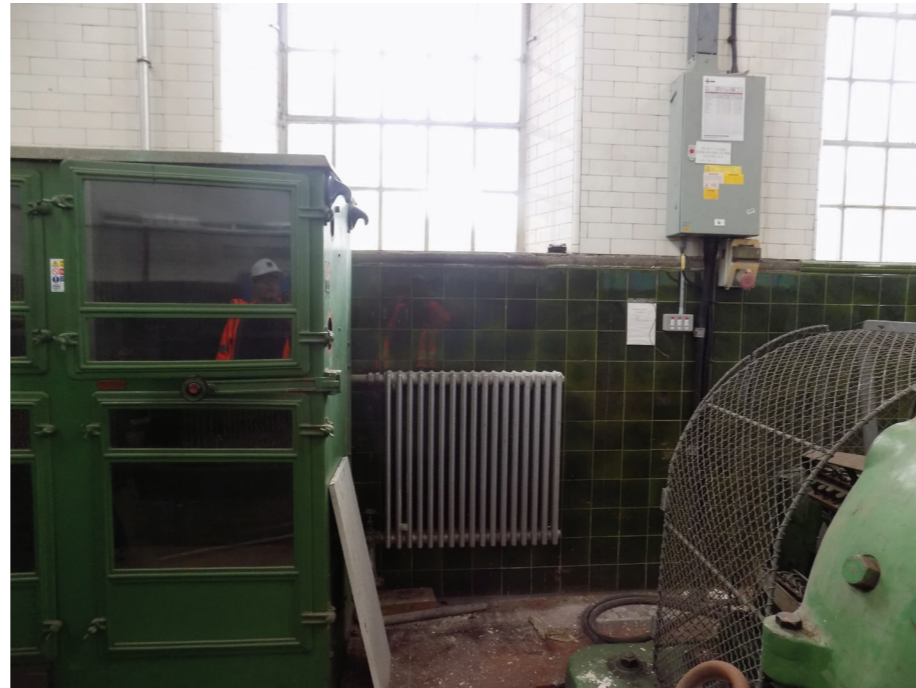
Figure 7: 1932 cast-iron radiator, Ruston & Ward Engine House (low significance)
