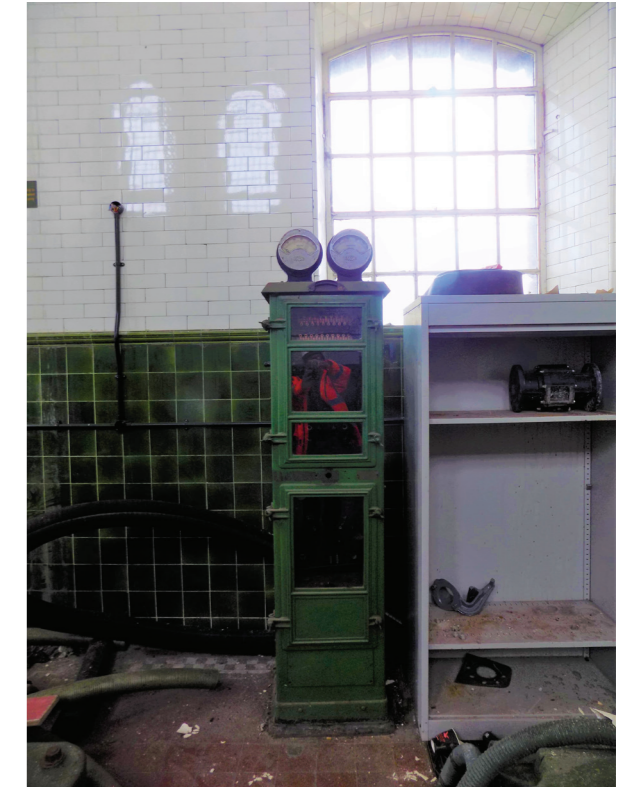
Figure 4: Control Cabinet for 1932 Harland electric centrifugal pumps, Ruston & Ward Engine House (low to medium significance)
