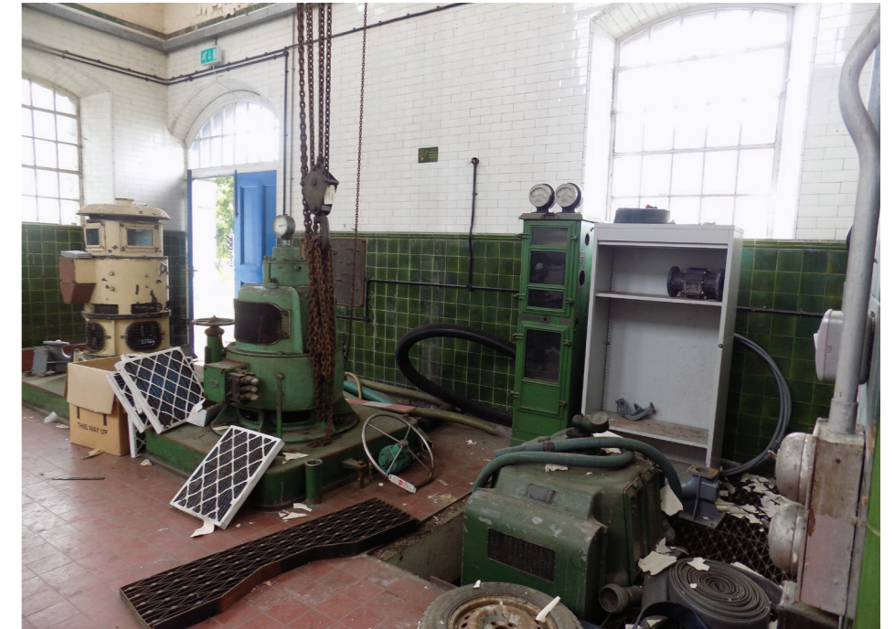
Figure 8: Three DC motors (two 1932 Harland plus one W H Allen replacement) driving centrifugal pumps down the historic Bull wells, Ruston & Ward Engine House (low to medium significance)
