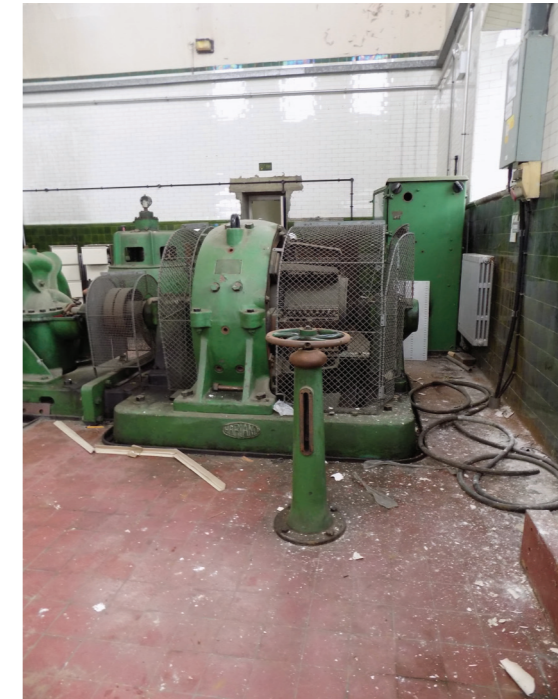
Figure 26: Valve control standard, 1932 Harland twin impeller electric centrifugal pump set, Ruston & Ward Engine House (low to medium significance)
