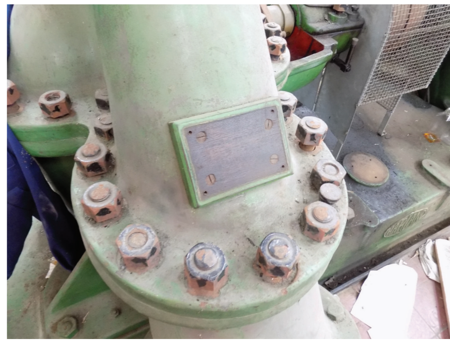
Figure 23: Detail of removed brass plate, 1932 Harland twin impeller electric centrifugal pump set, Ruston & Ward Engine House (low to medium significance)
