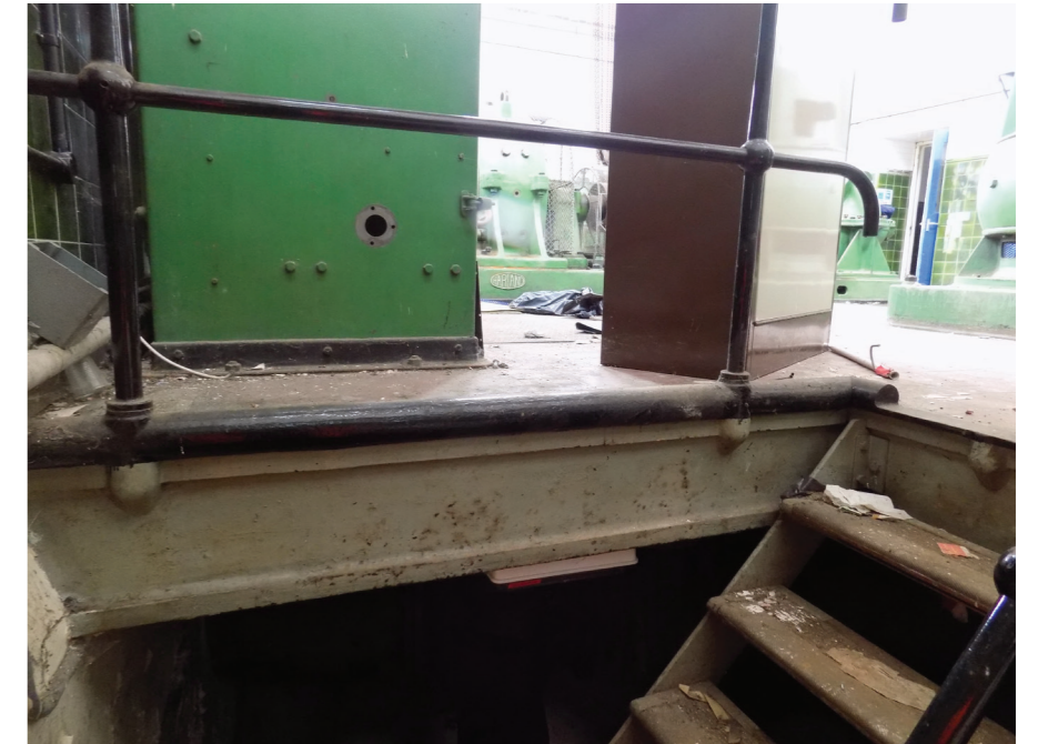
Figure 15: Reused cast iron beam incorporated in ground floor slab of Ruston & Ward Engine House (low significance)
