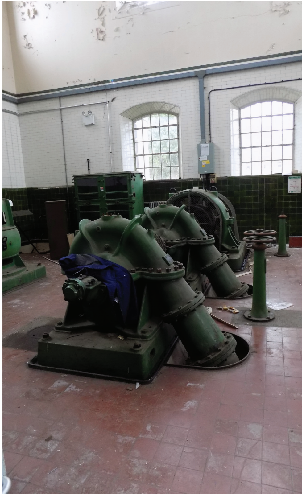
Figure 19: 1932 Harland twin impeller electric centrifugal pump set, Ruston & Ward Engine House (low to medium significance)
