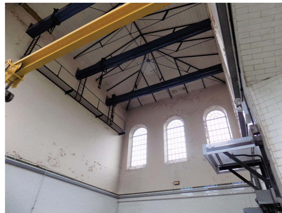
Figure 27: Primary lifting beams (3 of, for three Bull engines and later DC motors), Ruston & Ward Engine House (high significance)
