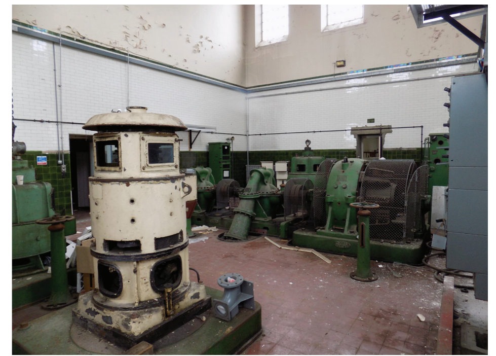
Figure 22: 1932 Harland twin impeller electric centrifugal pump set and WH Allen replacement DC motor, Ruston & Ward Engine House (low to medium significance)
