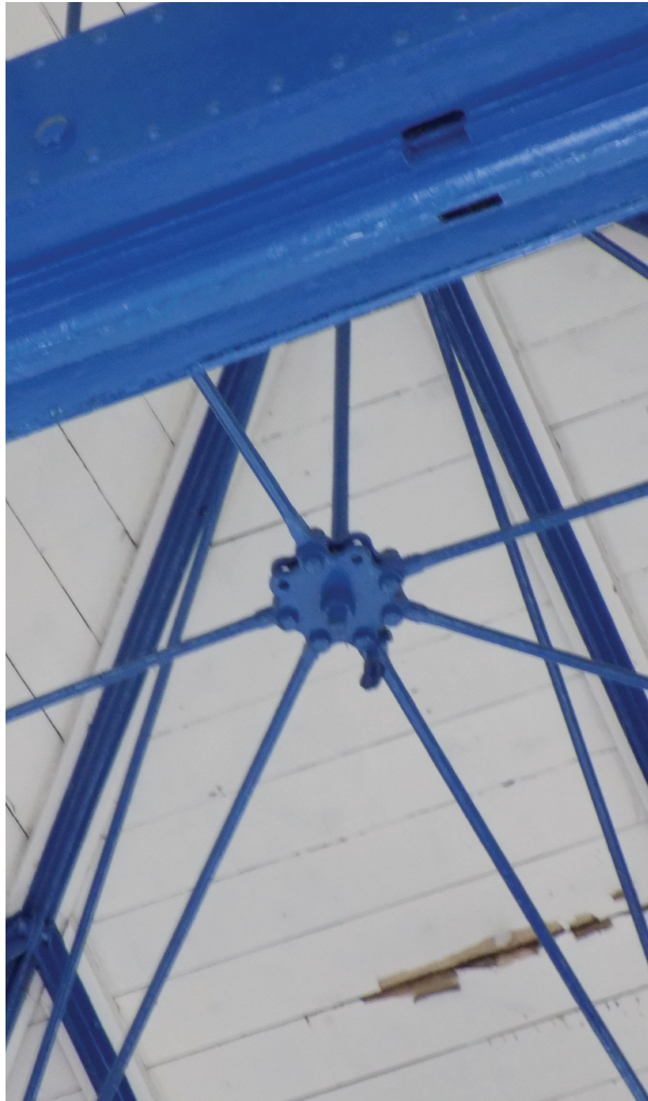
Figure 24: Detail of boss of primary wrought-iron roof (radial ties), Ruston & Ward Engine House (medium significance)
