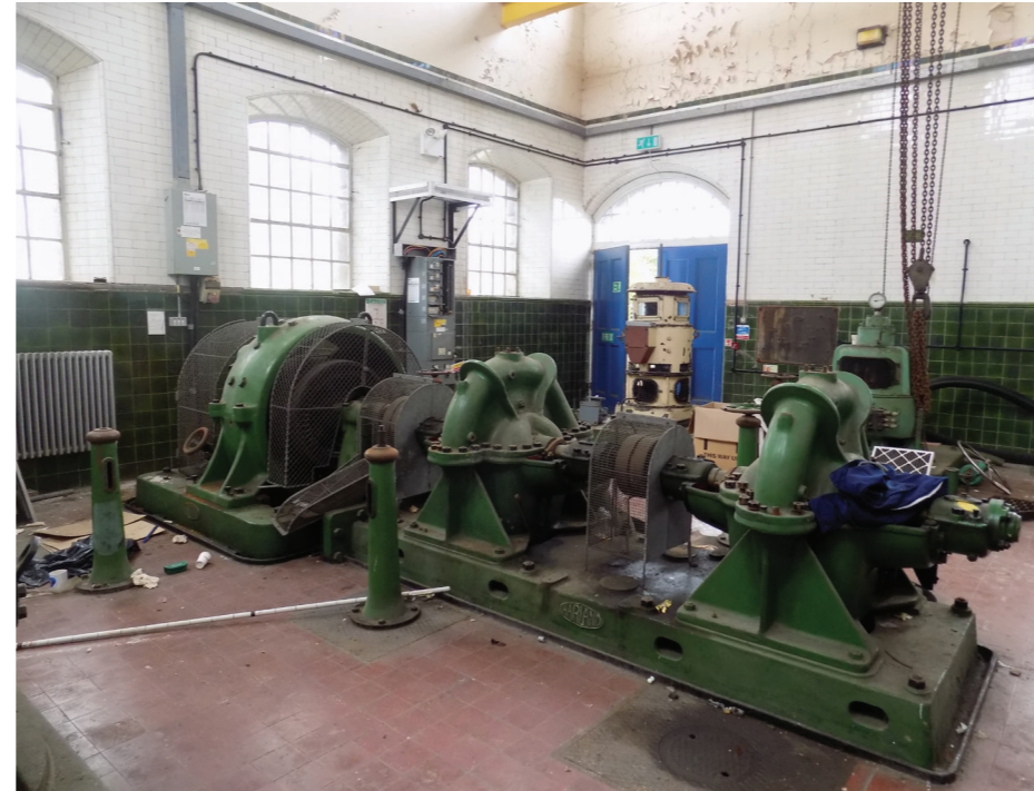
Figure 20: 1932 Harland twin impeller electric centrifugal pump set, Ruston & Ward Engine House (low to medium significance)
