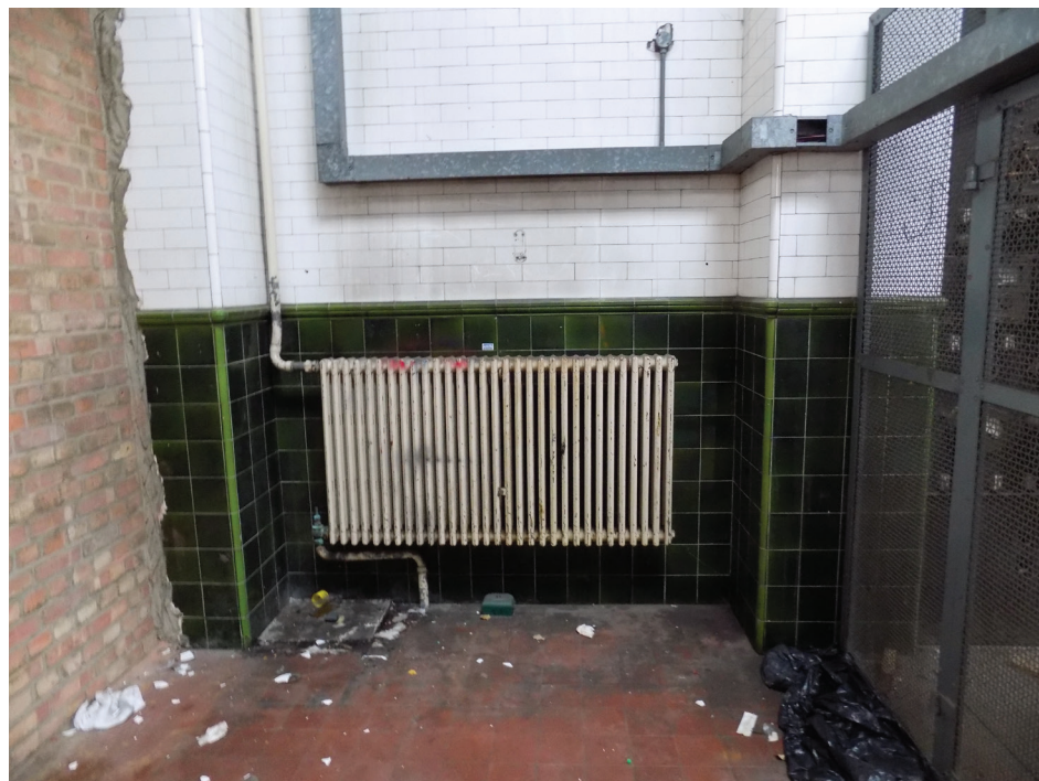
Figure 39: 1932 cast-iron radiator, former Ruston engine house (originally Sheffield's Boiler House) (low significance)
