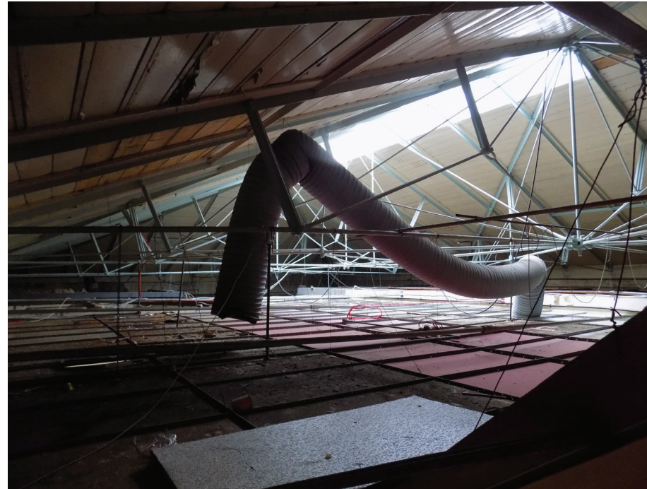
Figure 52: View of primary wrought-iron roof (radial ties), Ruston & Ward Former Boiler House (medium significance)
