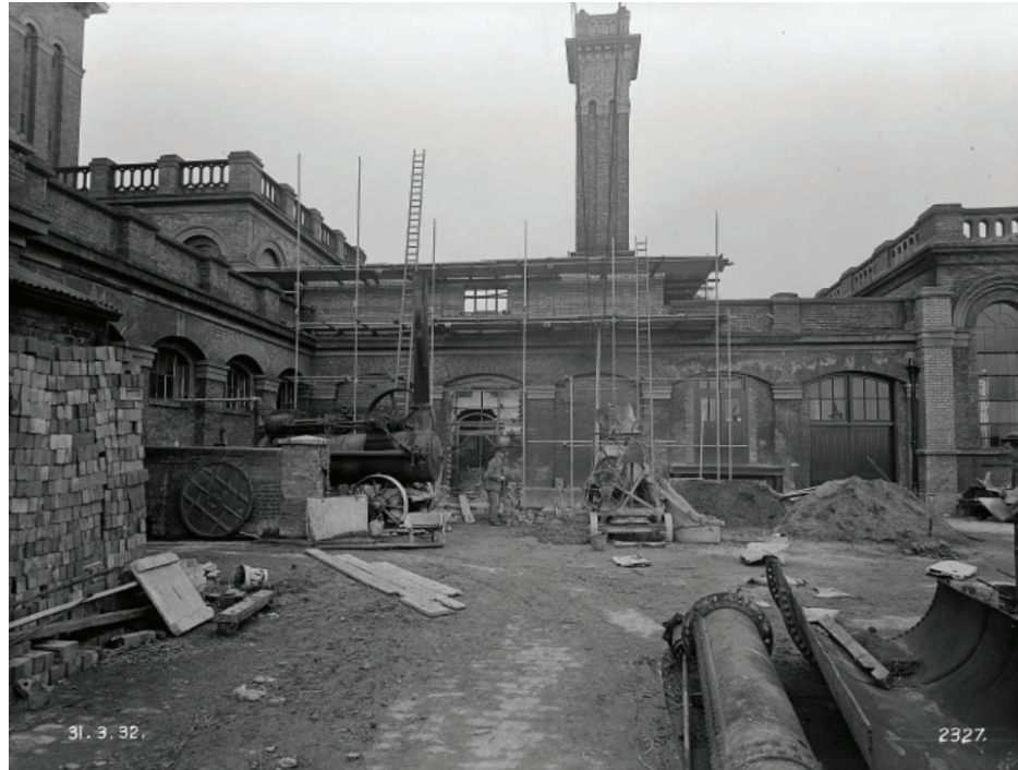
Figure 47: Ruston & Ward Former Ruston Engine House: Raising of walls of former Sheffield's boiler house and erection of new roof, during 1932 conversion for Ruston & Hornsby diesel generator set
