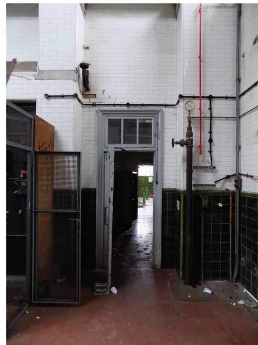
Figure 38: 1932 door and tiles, former Ruston engine house (originally Sheffield's Boiler House) (medium significance)
