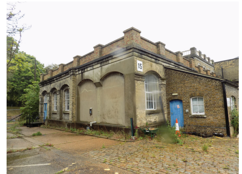
Figure 74: West end of the Former Boiler House, showing cement patched area marking the location of lost bay
