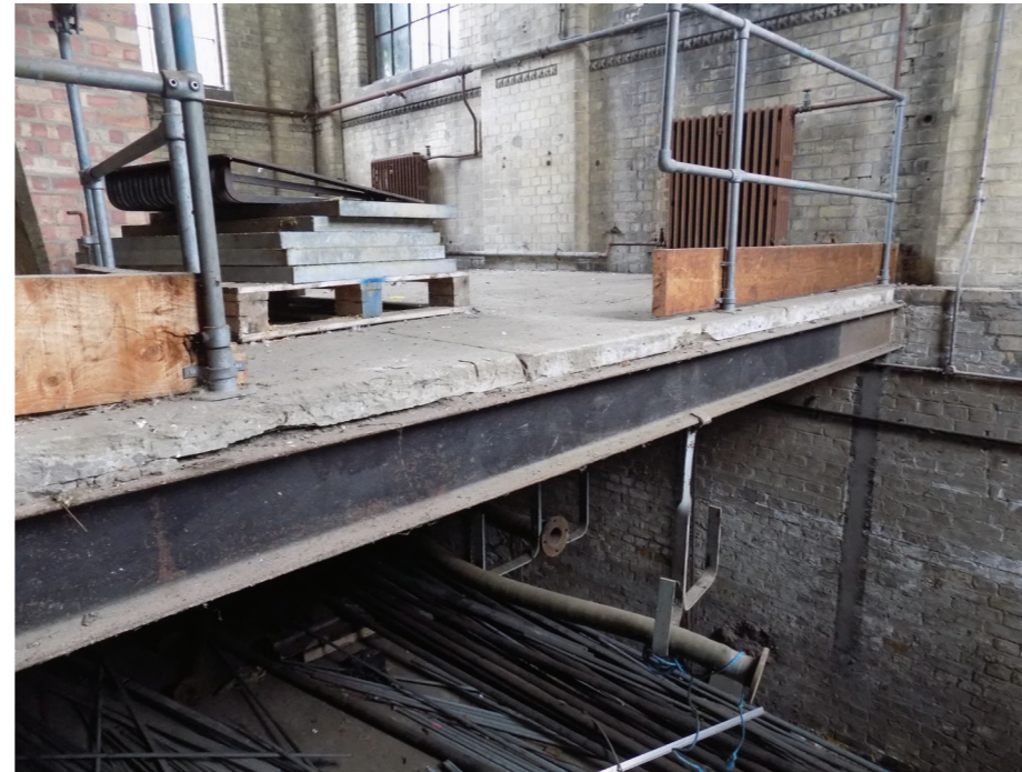
Figure 80: Intermediate floor of York slabs on rolled iron or steel joists (high significance)
