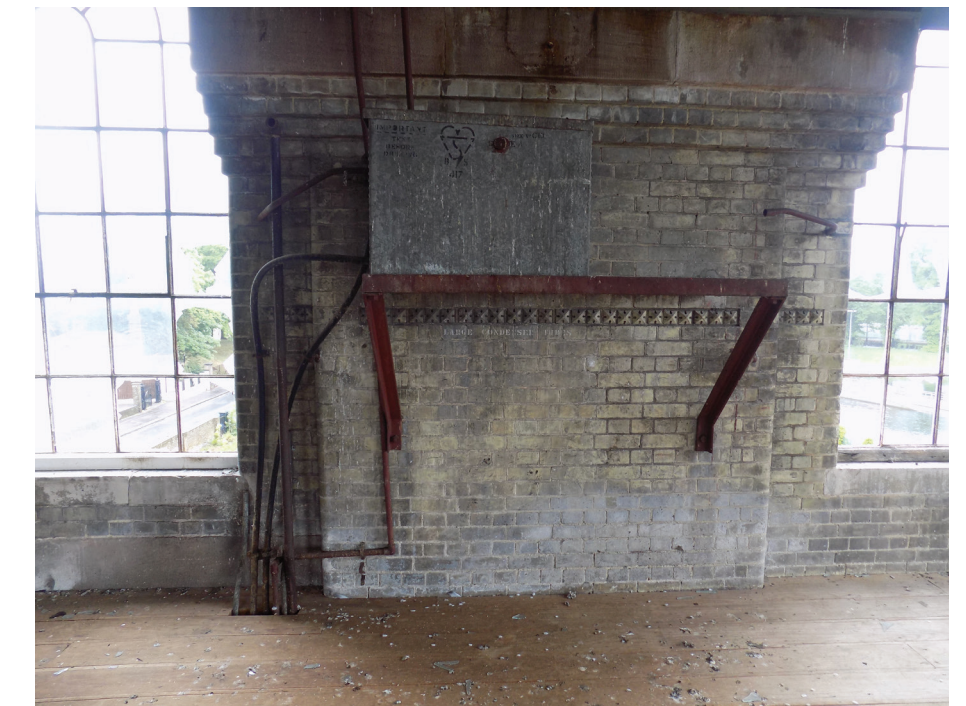
Figures 100: Header tank on welded steel supports (no significance)
