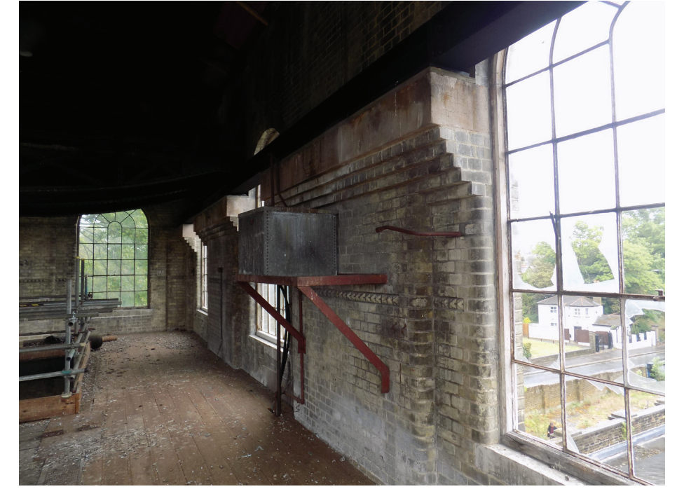
Figures 99: Header tank on welded steel supports (no significance)
