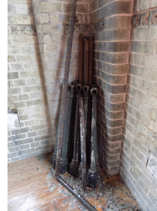
Figures 104: Displaced cast-iron handrail balusters (high significance)
