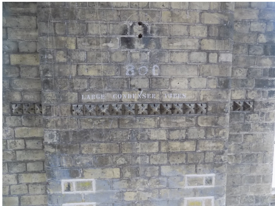
Figure 108: Stencilled "Large Condenser Tubes" (one of two) (high significance)
