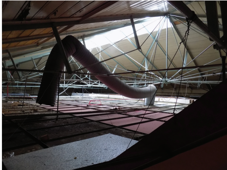
Figure 114: General view of primary wrought-iron boiler house roof with radial ties and modern suspended ceiling (medium significance)
