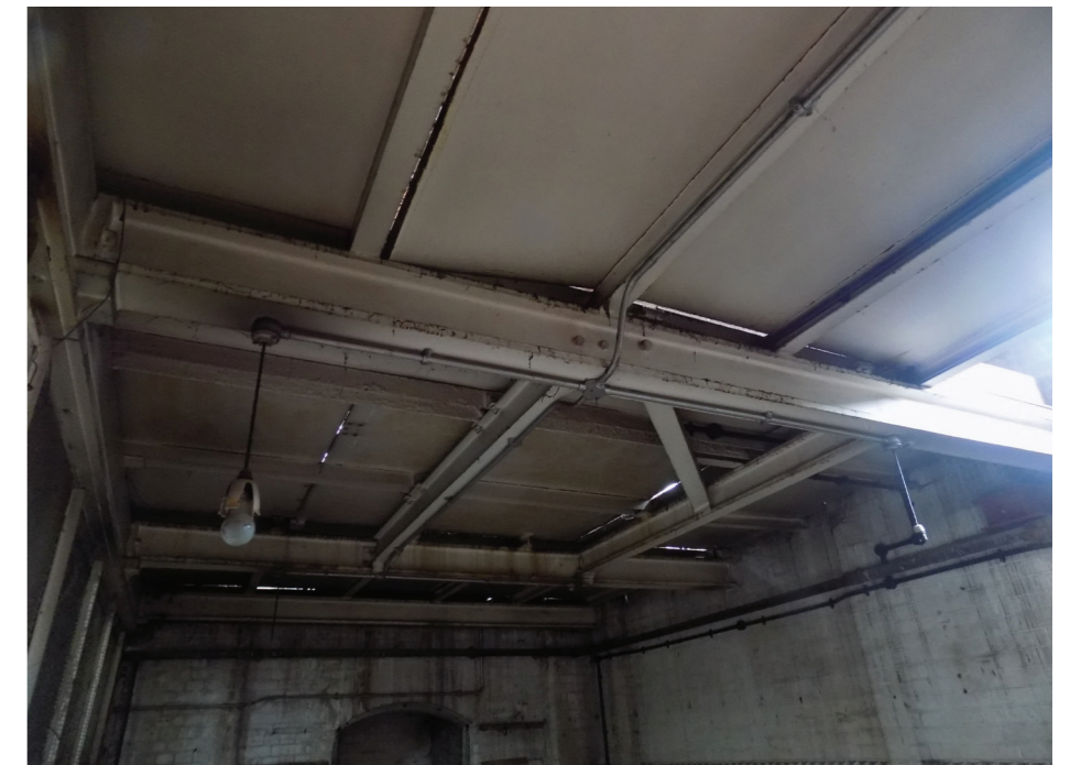
Figure 106: Beam loft floor and supporting joists from beneath (high significance) (steel sheet cladding of no significance)
