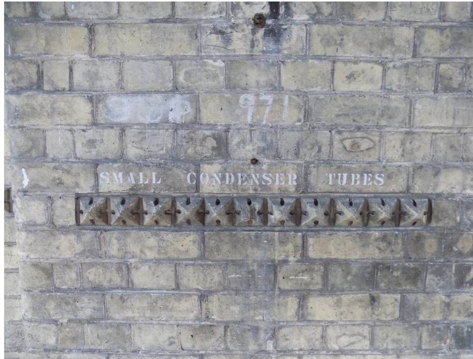
Figure 102: Stencilled "Small Condenser Tubes" (one of two) (high significance)
