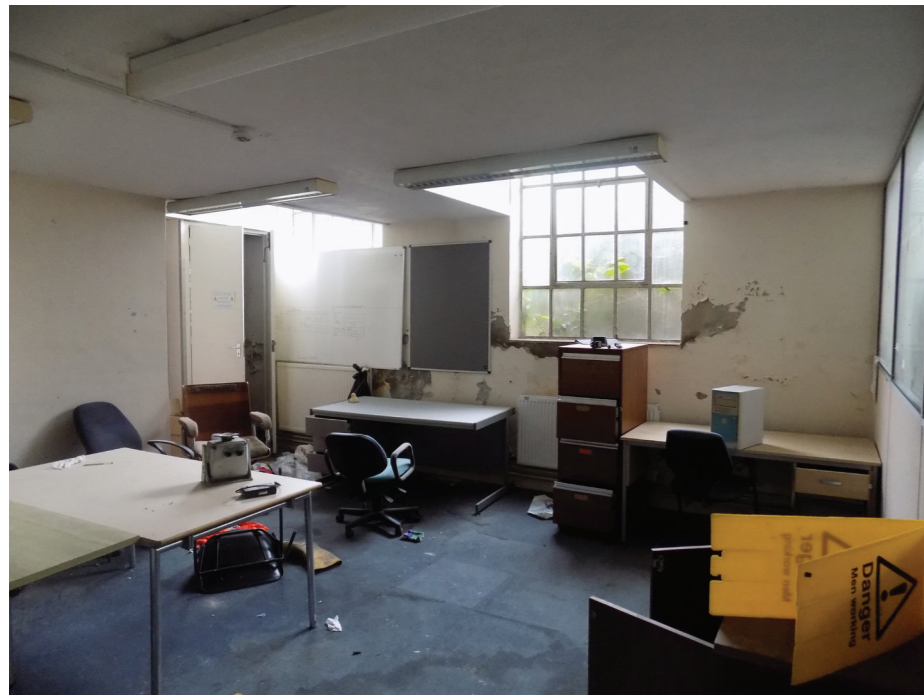
Figure 113: 1930s Crittall-type steel casement windows in north wall of Former Boiler House (wall originally blind) (low significance)
