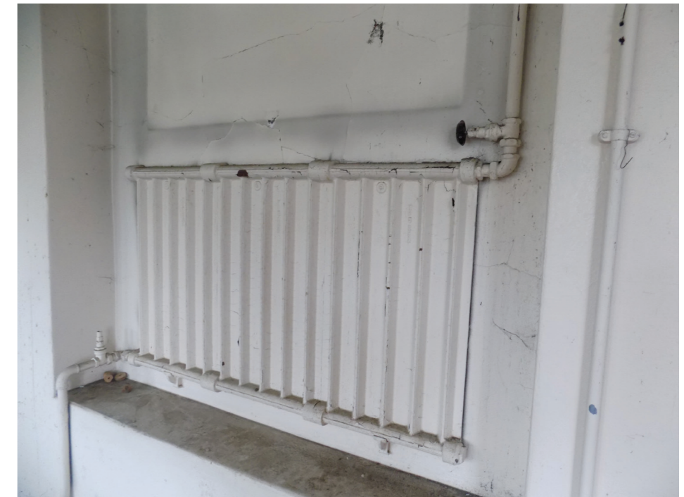
Figures 111: 1930s flat panel cast-iron radiators in 19th-century extension south of Beam Engine House (low significance)
