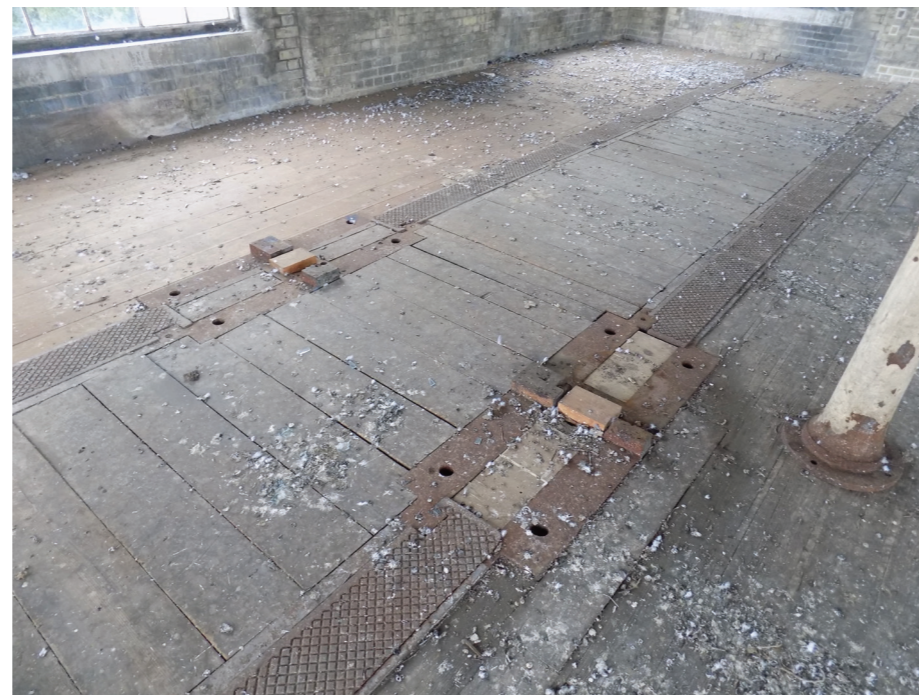
Figure 107: Beam loft floor showing spring beams and trunnion bearing support (high significance) and later infill to beam openings (no significance)
