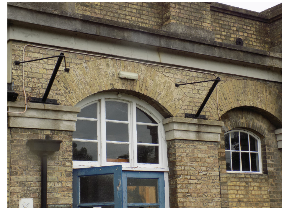
Figure 129: Karslake Boiler House, South Elevation. Timber framed toplight window, likely a post-war replacement of very low interest.
