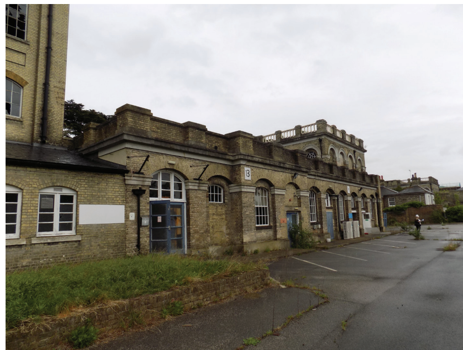
Figure 130: Karslake Boiler House, South Elevation, between Karslake West (RHS) and Karslake East (LHS)
