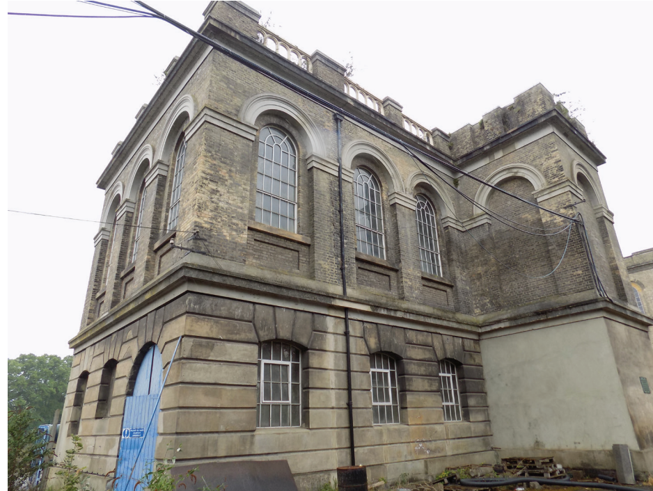
Figure 118: Karslake East, original Bull Engine House with cement repair to base of former pump head tower.
