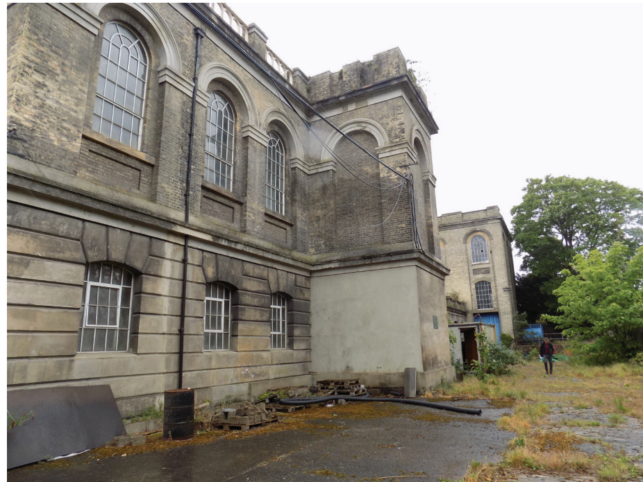
Figure 122: Karslake East, expressed as two-storey building, in and Karslake West, expressed as a three-storey building which distinguishes the type of engines each building was purpose built to house.
