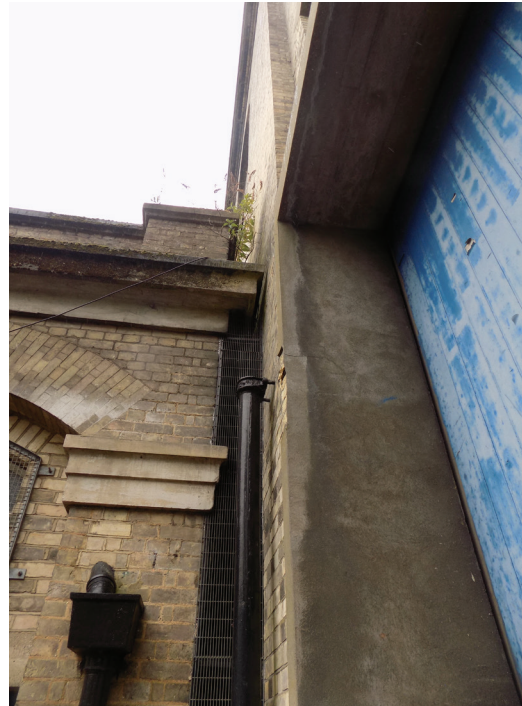
Figure 125: Metal rain water down pipe at corner of Karlast Boiler House and Karslake West Engine House.
