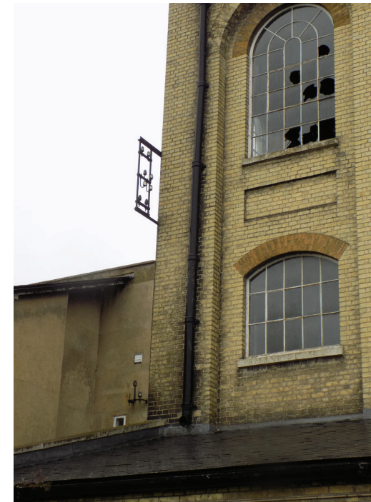
Figure 127: Karslake West, showing arrangement and hierarchy of two levels above ground level. 19thC windows remain in situ.
