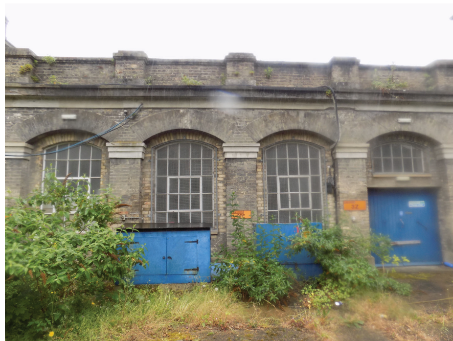
Figure 124: Karslake Boiler House with windows established in 1930s when the boilers were removed and the buildings were converted to office space.
