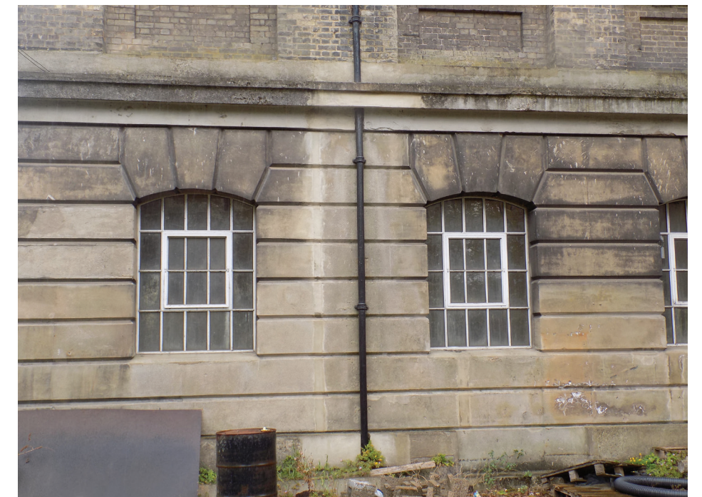
Figure 120: Karslake East, original Bull Engine House with 1930s crittal-type windows installed at ground floor level.
